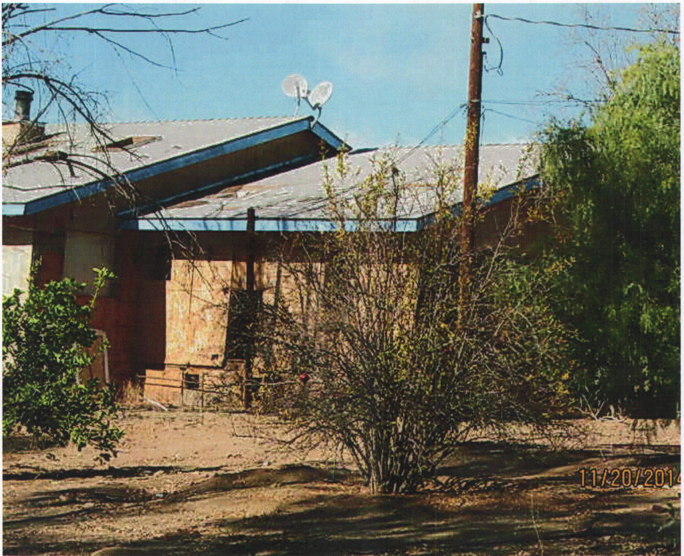
Substandard Structures Remain. Lpadilla - 11/20/2014
