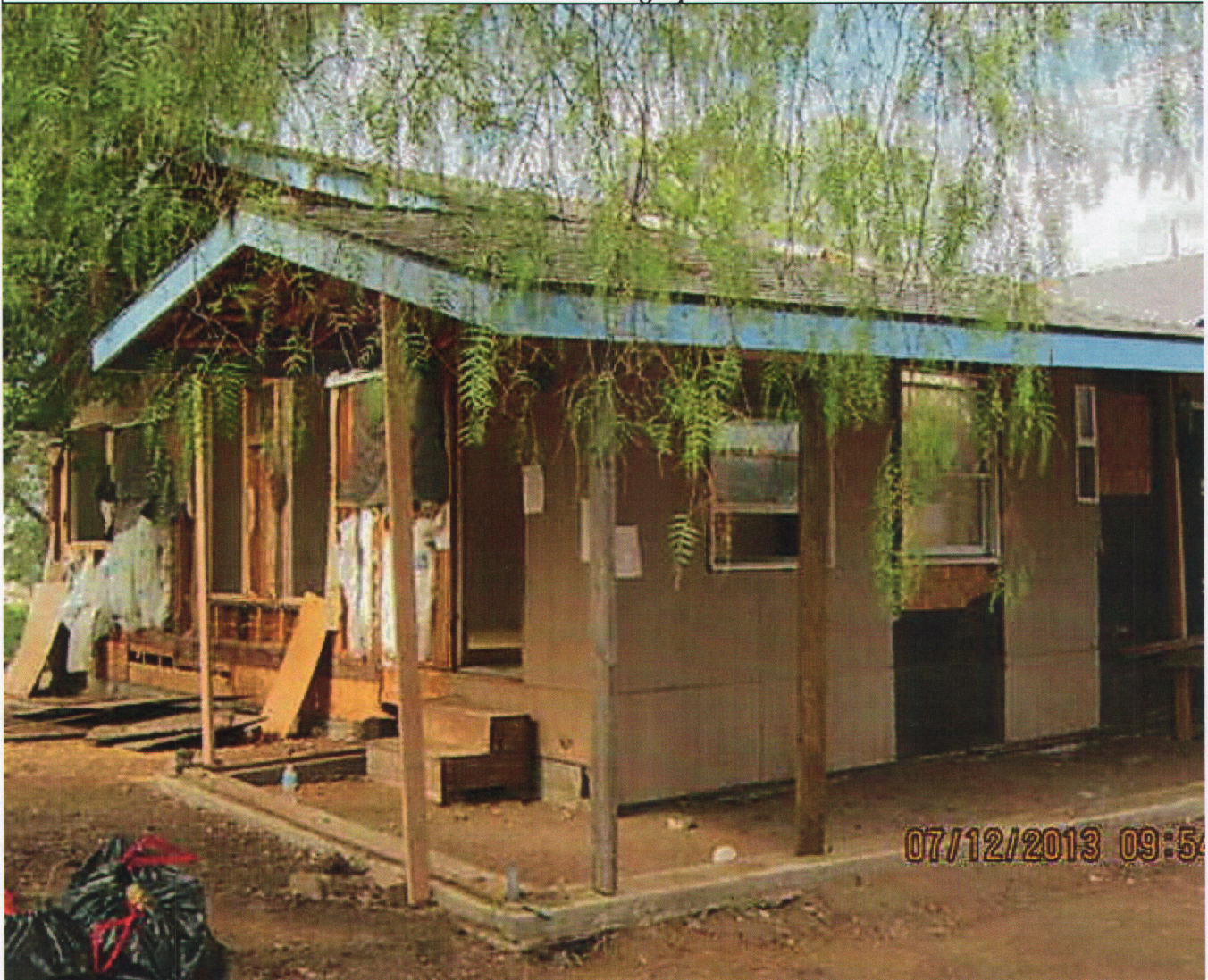
E. Torres; SS#1 dwelling/defects- 6, 9, 10, 12, 13, 14, 17 - 07/12/2013
