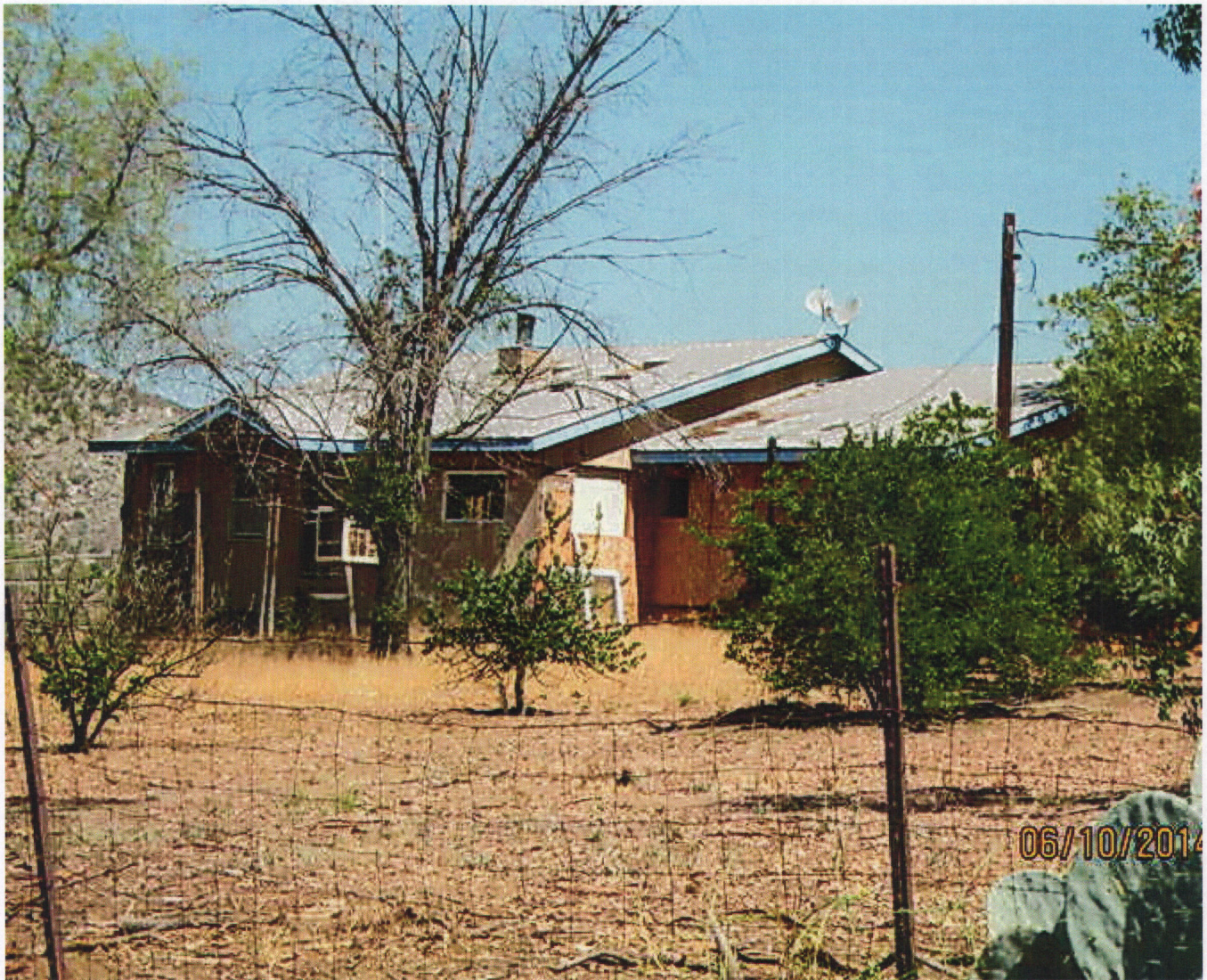
Substandard Structures. Lpadilla - 06/10/2014
