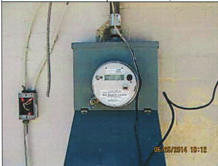
Photo taken on the parcel (electric meter) D Jurden, CET
