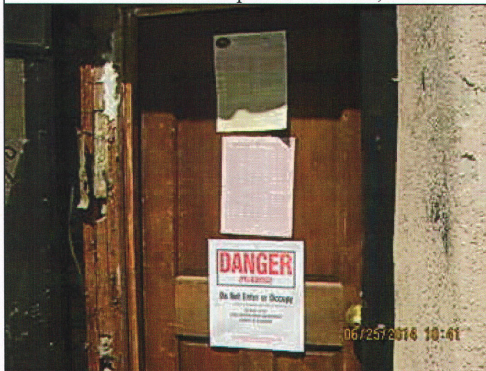
Photo taken of the posting (acc structure) D Jurden, CET
