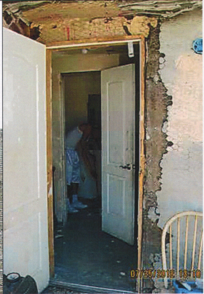
Substandard Structure 7/25/12 J. Cole
