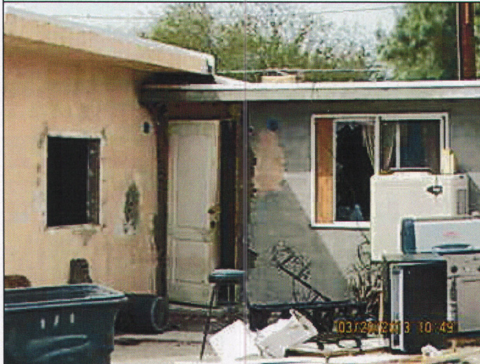
Substandard Structure 3/20/13 J. Cole
