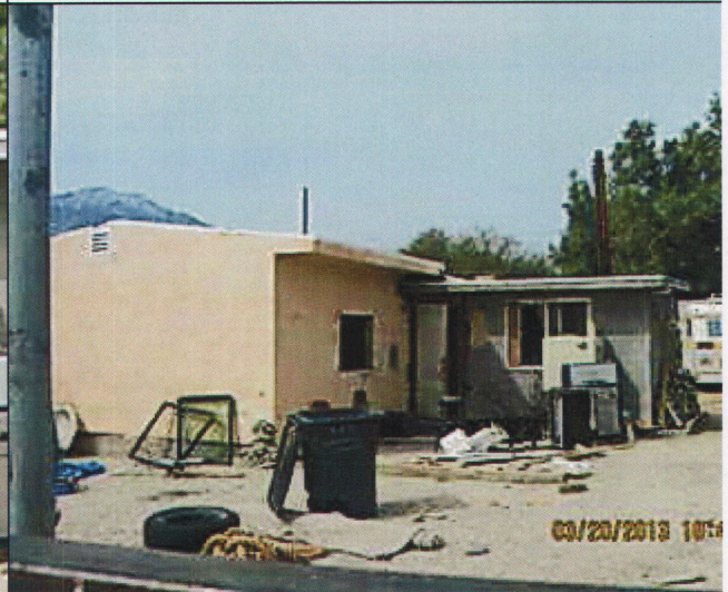
Substandard Structure 3/20/13 J. Cole
