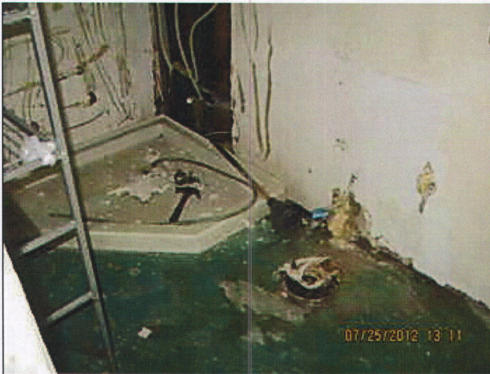
Substandard Structure 7/25/12 J. Cole
