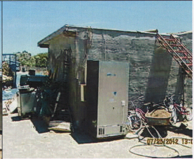
Substandard Structure 7/25/12 J. Cole
