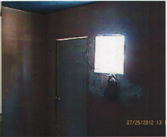
Substandard Structure 7/25/12 J. Cole
