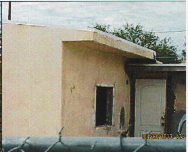
Substandard Structure 1/23/13 J. Cole
