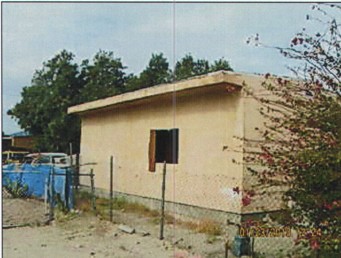
Substandard Structure 1/23/13 J. Cole
