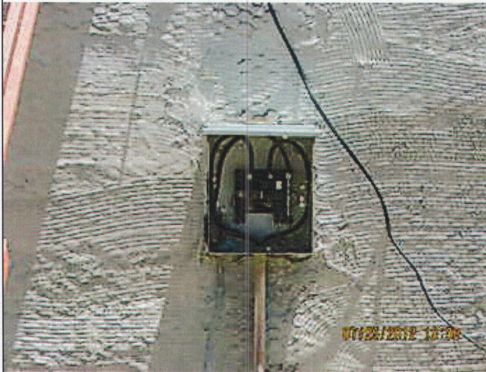
Substandard Structure 7/25/12 J. Cole
