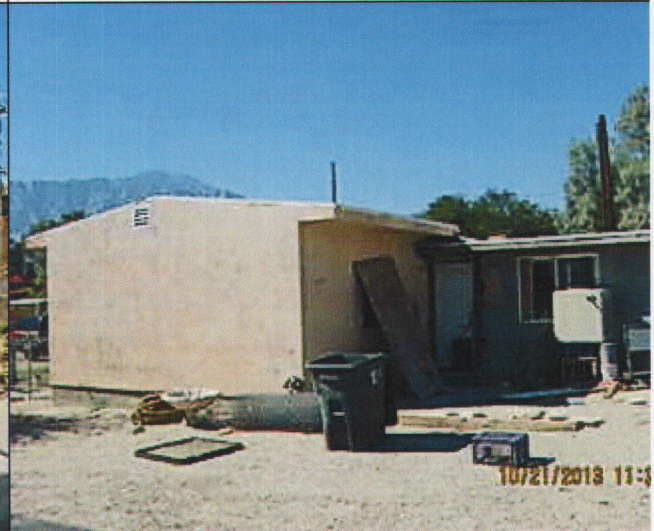
Substandard Structure 10/21/13 J. Cole
