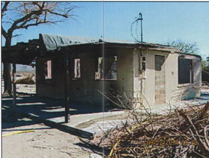
Substandard Structure and Rubbish Remain 9/12/14 J. Cole
