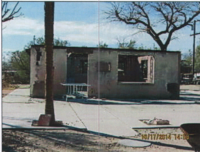
Substandard Structure and Rubbish Remain 10/17/14 J. Cole
