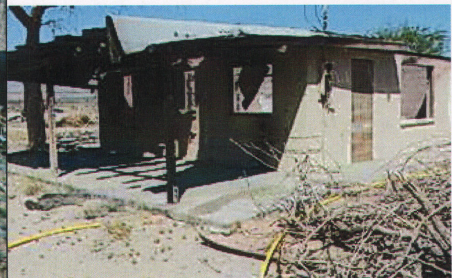
Substandard Structure 4/8/15 J. Cole
