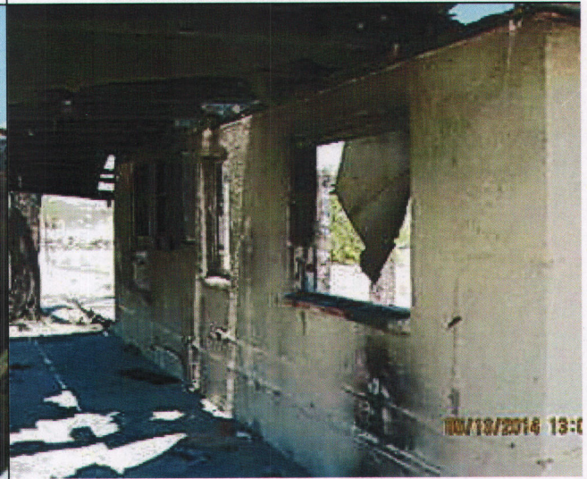
Substandard Structure 6/13/14 J. Cole
