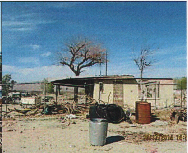
Substandard Structure and Rubbish Remain 10/17/14 J. Cole
