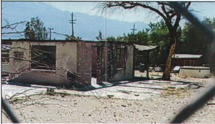
Substandard Structure 4/8/15 J. Cole
