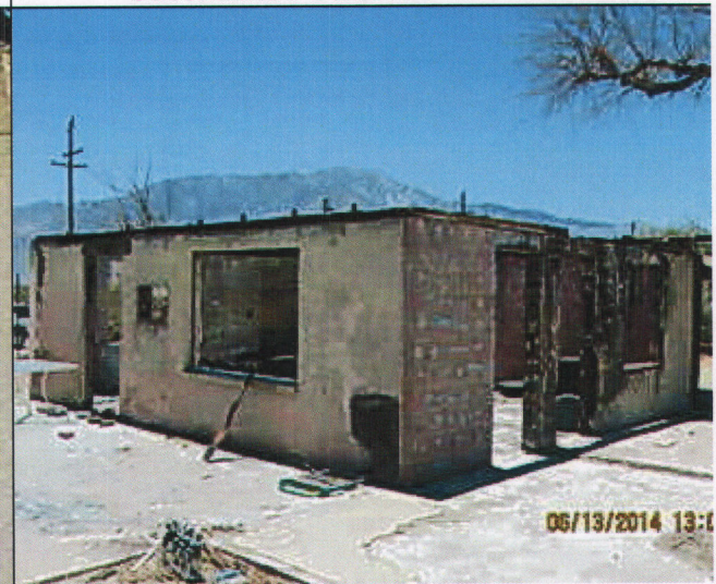
Substandard Structure 6/13/14 J. Cole
