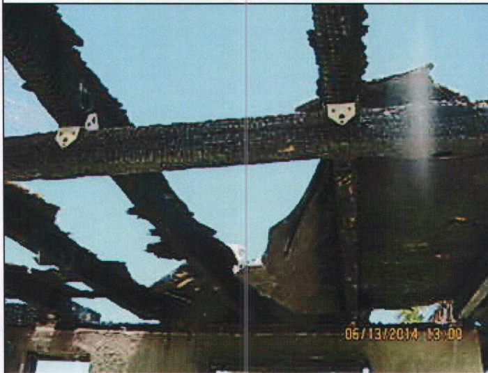
Substandard Structure 6/13/14 J. Cole
