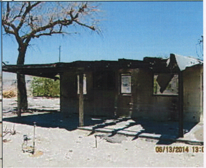
Substandard Structure 6/13/14 J. Cole
