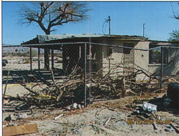
Substandard Structure and Rubbish Remain 9/12/14 J. Cole
