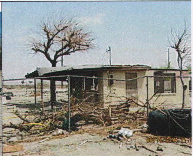
Substandard Structure and Rubbish Remain 8/18/ Cole
