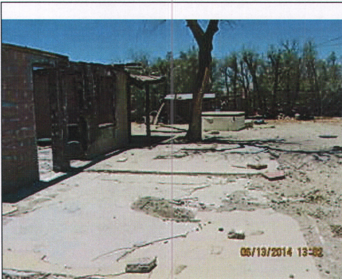
Substandard Structure 6/13/14 J. Cole
