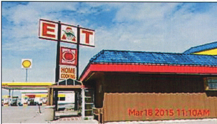
E. Torres; substandard structure continues to deteriorate
