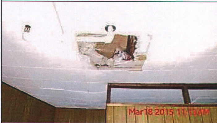
E. Torres; substandard structure continues to deteriorate
