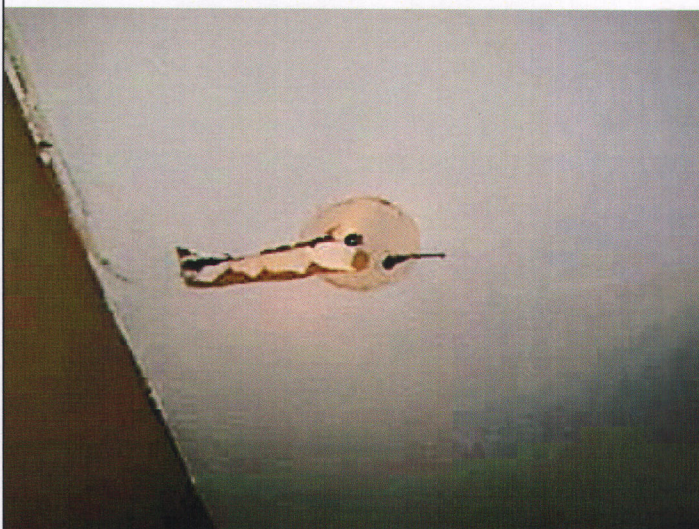
-09/26/14 - Initial Inspection SSST Verified - NOD#
