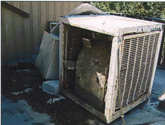
-09/26/14 - Initial Inspection SSST Verified - NOD# 14,17 - Pike
