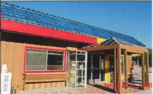
E. Torres; structure remains in substandard condition
