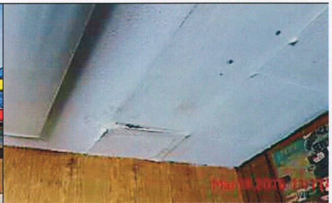
E. Torres; substandard structure continues to deteriorate
