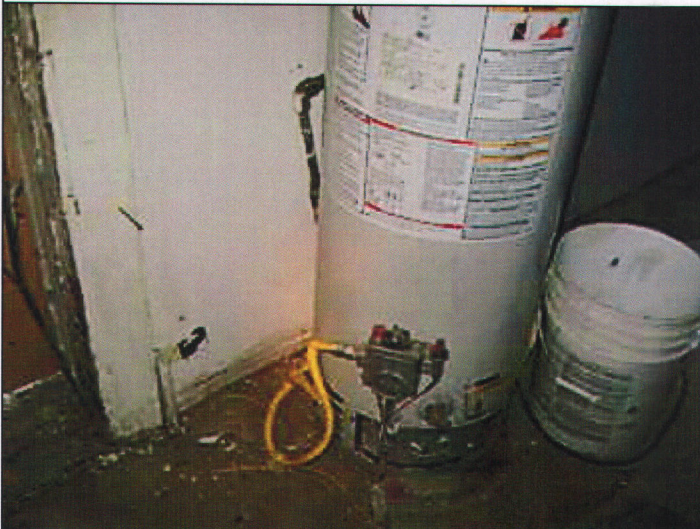
-09/26/14 - Initial Inspection SSST Verified - NOD# 1,2 - Pike
