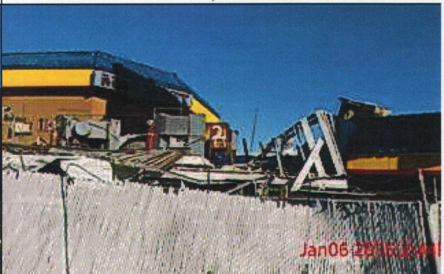
-E. Torres; structure remains in substandard condition
