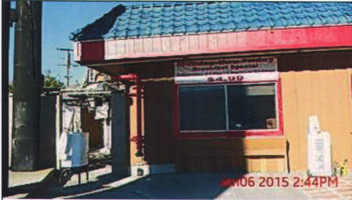
-E. Torres; structure remains in substandard condition
