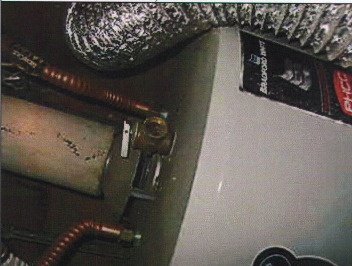
09/26/14 - Initial Inspection SSST Verified - NOD# 1,2 - Pike
