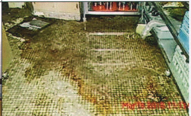
E. Torres; substandard structure continues to deteriorate
