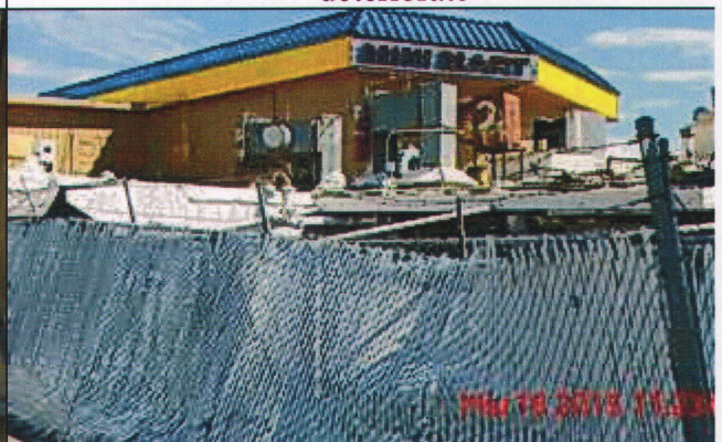
E. Torres; substandard structure continues to deteriorate
