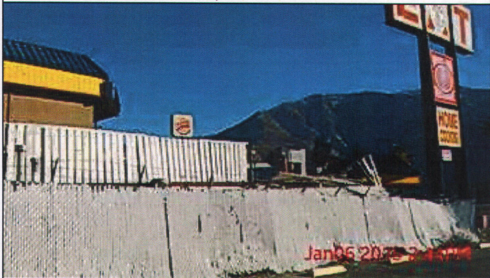
E. Torres; structure remains in substandard condition
