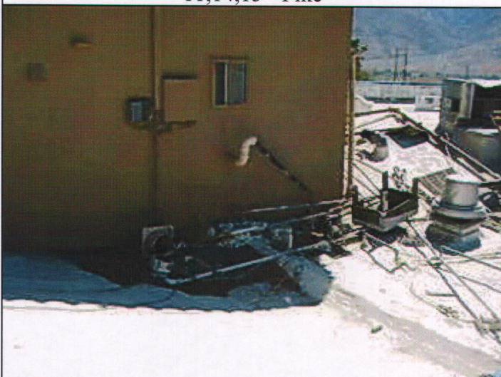
-09/26/14 - Initial Inspection SSST Verified - NOD# 14,17 - Pike
