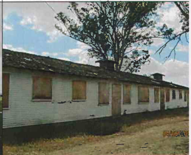
Property remains in violation. Lpadilla
