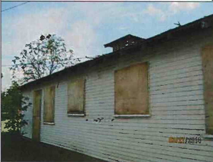
SUBSTANDARD STRUCTURE. LPADILLA
