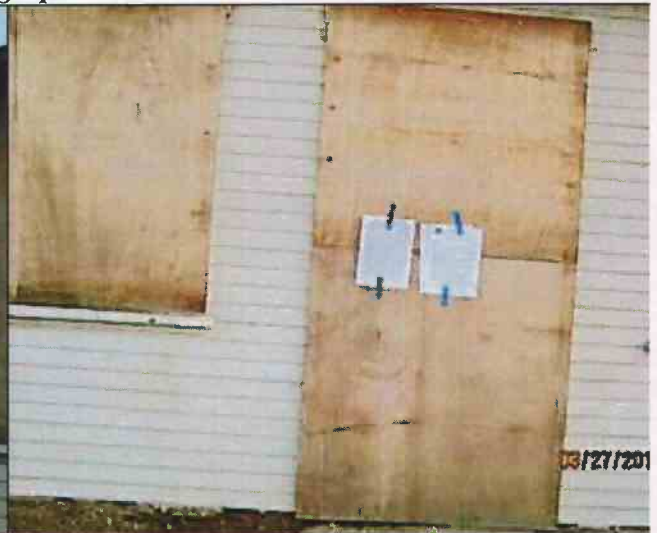
SUBSTANDARD STRUCTURE. LPADILLA
