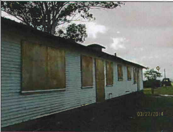
SUBSTANDARD STRUCTURE. LPADILLA
