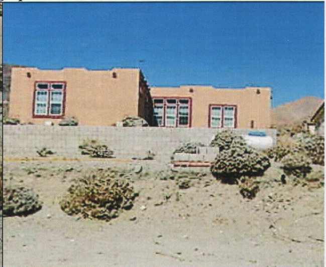
09/28/12 - Accumulated Rubbish - Pike
