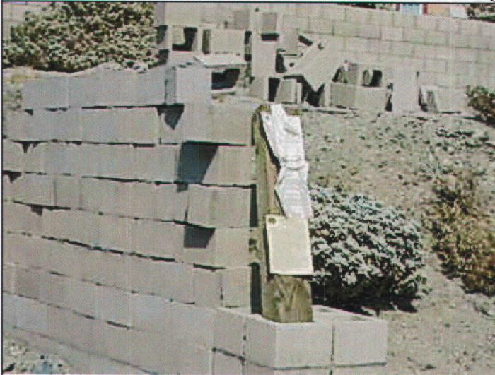
09/28/12 - Accumulated Rubbish - Pike
