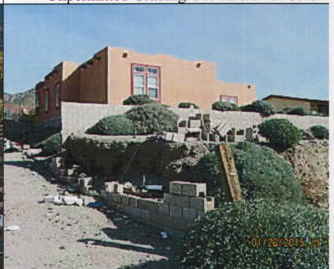
Unpermitted Grading/Cut 1/28/15 J. Cole
