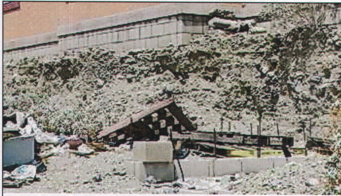
Unstable Foundation Along the West Side of the Structure 6/29/15 J. Cole
