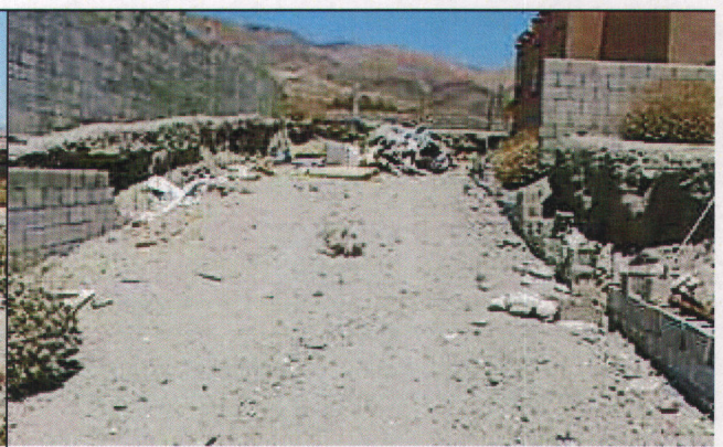
Unpermitted Grading 7/9/15 J. Cole
