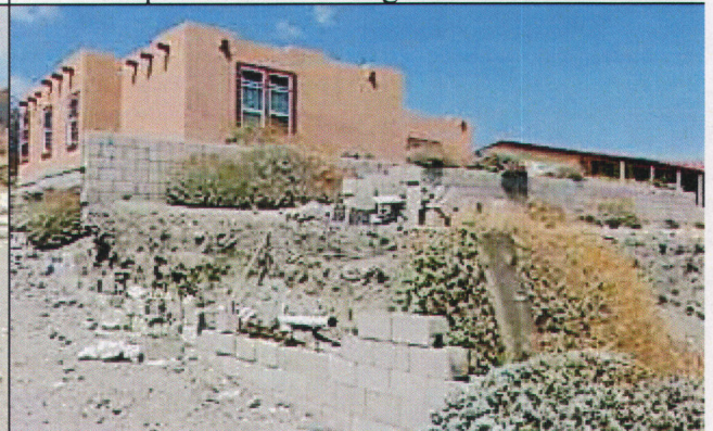
Unpermitted Grading/Cut 5/7/15 J. Cole
