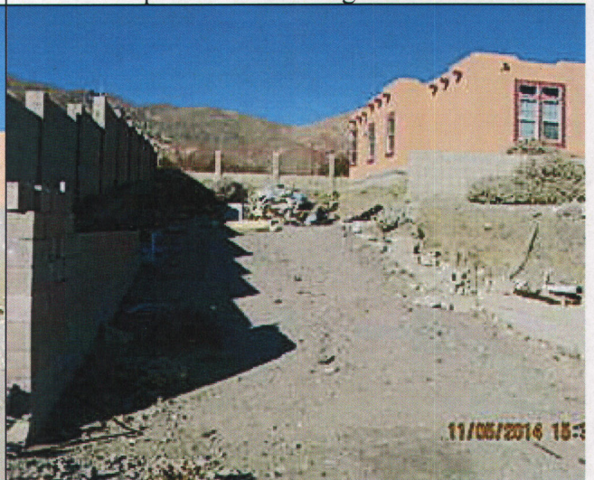
Unpermitted Grading/Cut 11/5/14 J. Cole
