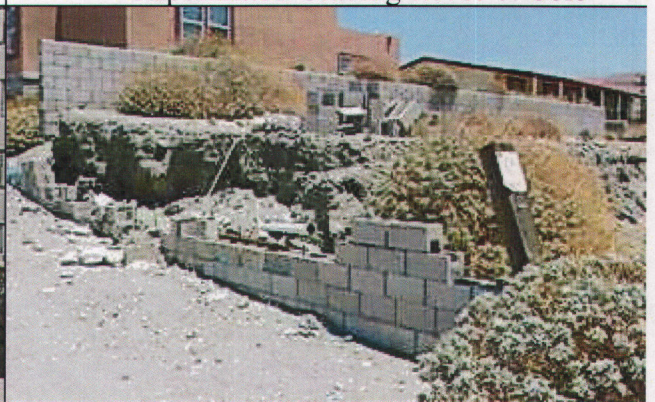
Unpermitted Grading 7/9/15 J. Cole
