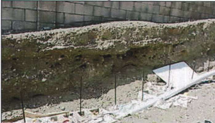
Unpermitted Grading/Cut 3/18/15 J. Cole
