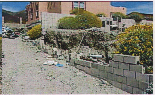
Unpermitted Grading/Cut 3/18/15 J. Cole
