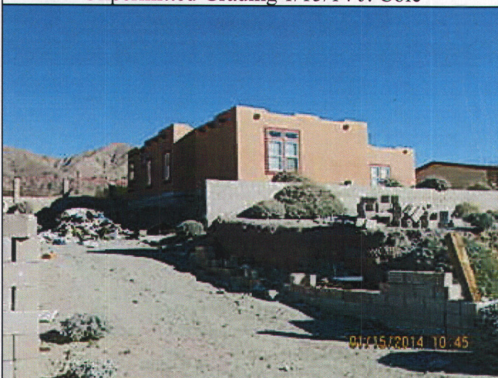
Unpermitted Grading 1/15/14 J. Cole
