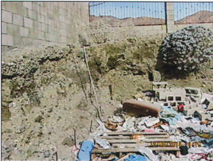
Unpermitted Grading/Cut 12/8/14 J. Cole
