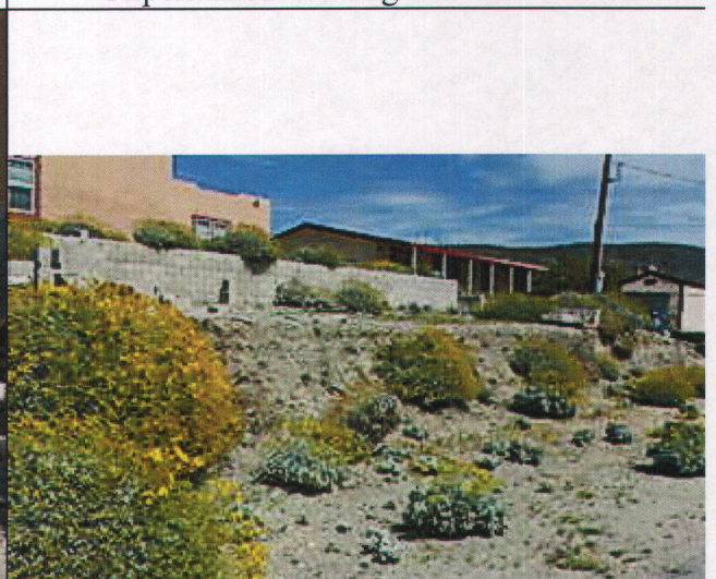
Unpermitted Grading/Cut 3/18/15 J. Cole
