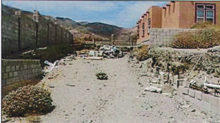
Unpermitted Grading/Cut 6/29/15 J. Cole
