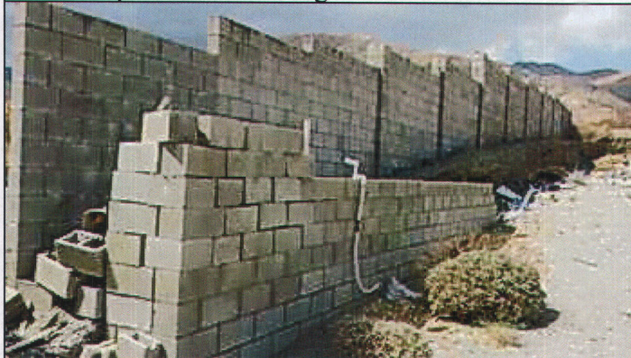
Unpermitted Grading/Cut 5/7/15 J. Cole
