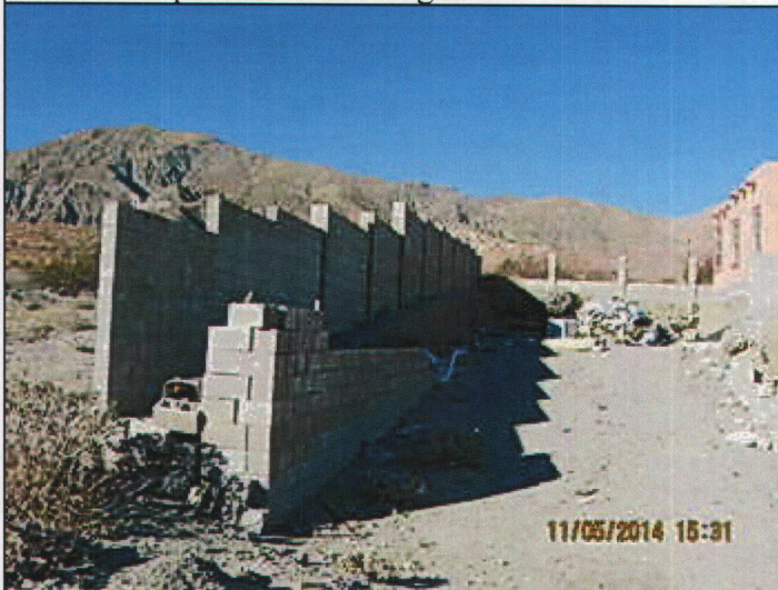
Unpermitted Grading/Cut 11/5/14 J. Cole
