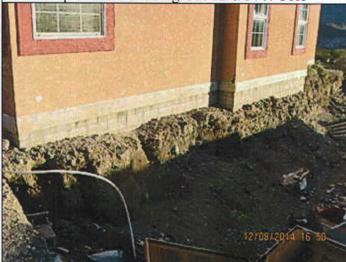
Unpermitted Grading/Cut 12/8/14 J. Cole
