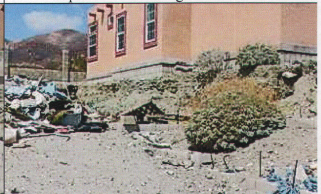
Unpermitted Grading/Cut 5/7/15 J. Cole
