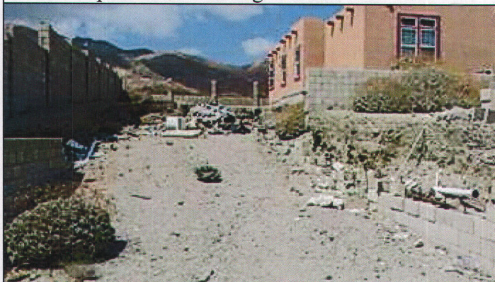
Unpermitted Grading/Cut 5/7/15 J. Cole
