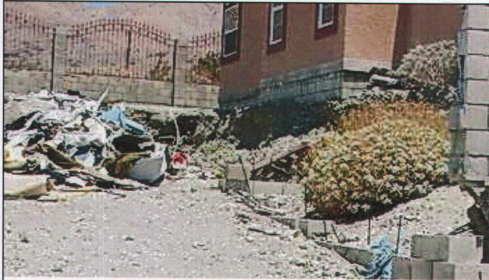
Unpermitted Grading 7/9/15 J. Cole
