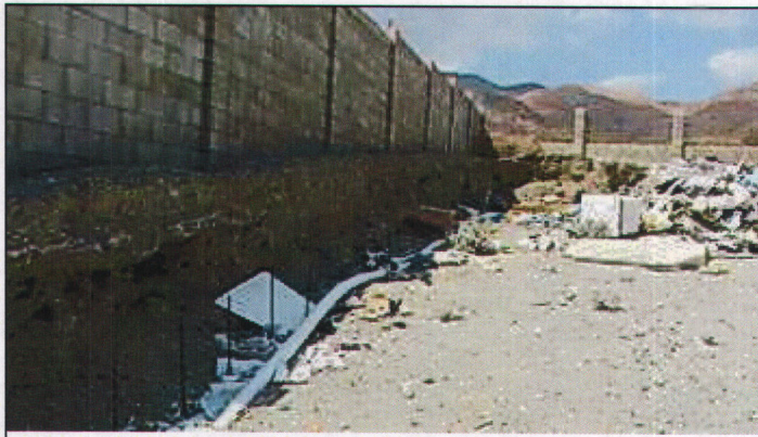
Unpermitted Grading/Cut 5/7/15 J. Cole
