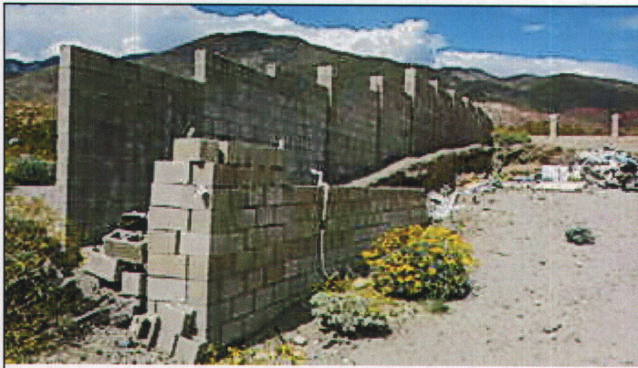
Unpermitted Grading/Cut 3/18/15 J. Cole
