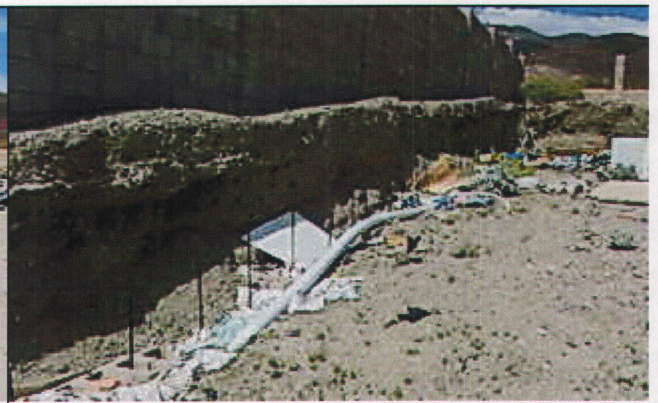
Unpermitted Grading/Cut 3/18/15 J. Cole
