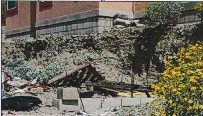
Unpermitted Grading/Cut 3/18/15 J. Cole
