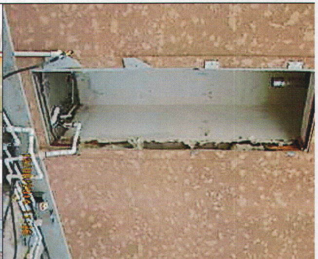
Missing Water Heater 12/8/14 J. Cole
