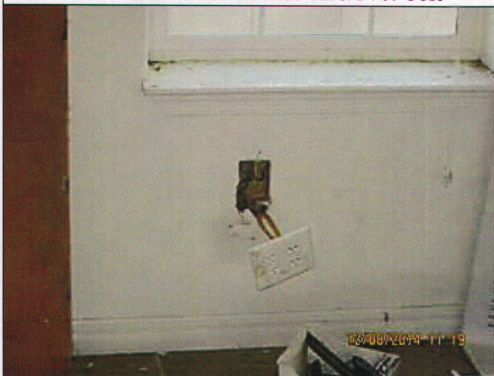
Hazardous Electrical 12/8/14 J. Cole
