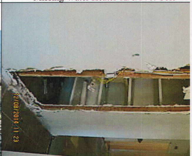
Hole in the Wall, Hazardous Electrical 12/8/14 J. Cole
