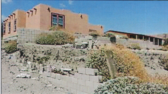
Substandard Structure 5/7/15 J. Cole
