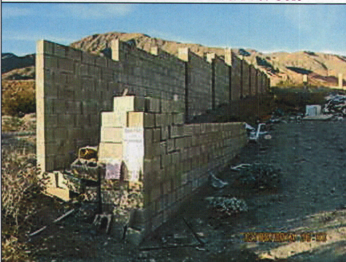
Substandard Block Wall 12/8/14 J. Cole
