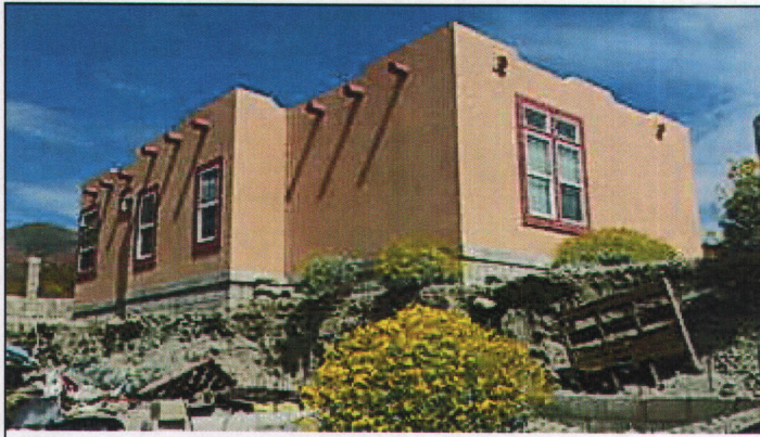
Substandard Structure 3/18/15 J. Cole
