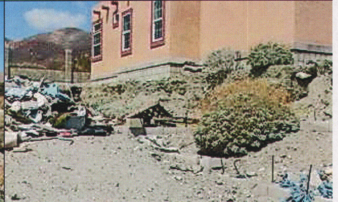
Substandard Structure 5/7/15 J. Cole
