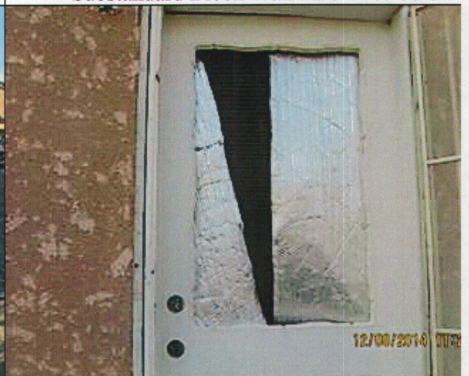
Damaged/Unsecured Rear Door 12/8/14 J. Col
