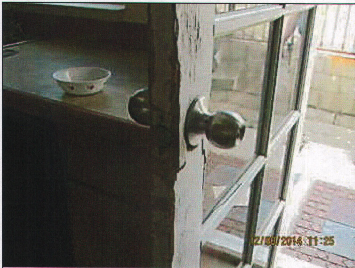
Damaged/Unsecured Rear Door 12/8/14 J. Cole
