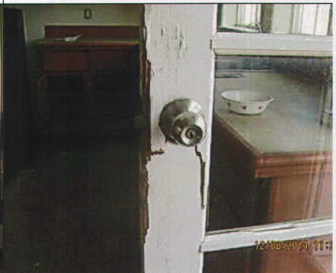
Damaged/Unsecured Rear Door 12/8/14 J. Col
