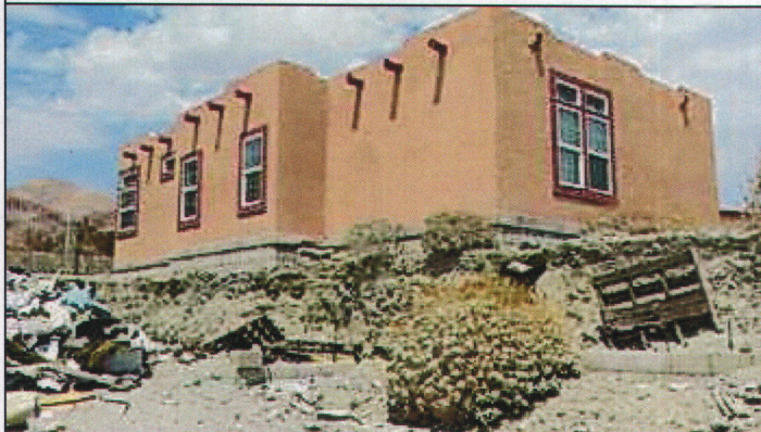
Substandard Structure 6/29/15 J. Cole
