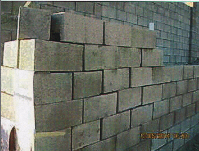
Substandard Block Wall 12/8/14 J. Cole
