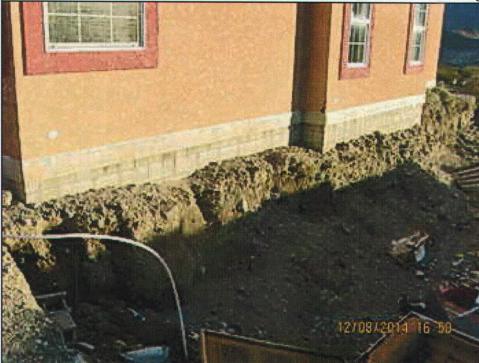
Deteriorated Foundation 12/8/14 J. Cole
