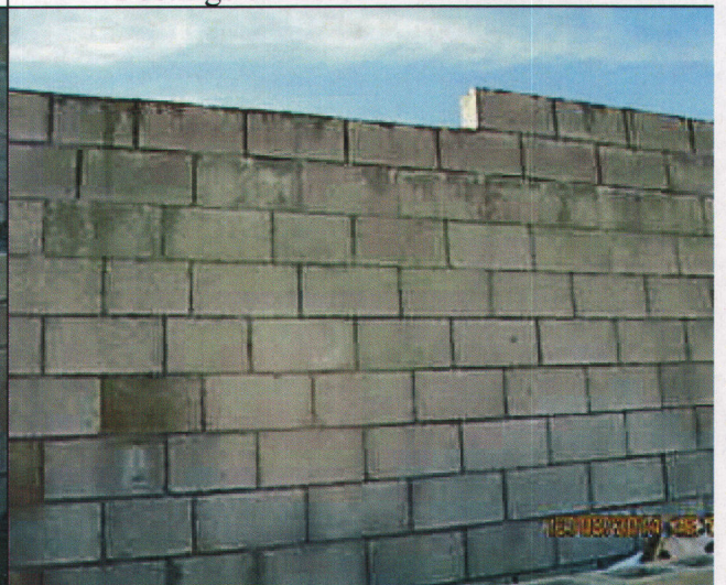
Substandard Block Wall 12/8/14 J. Cole
