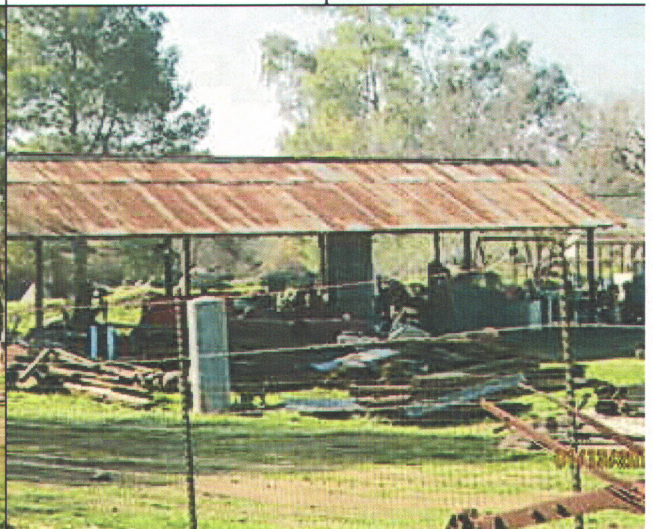
Accumulated Rubbish & Excessive Outside Storage. Lpadilla
