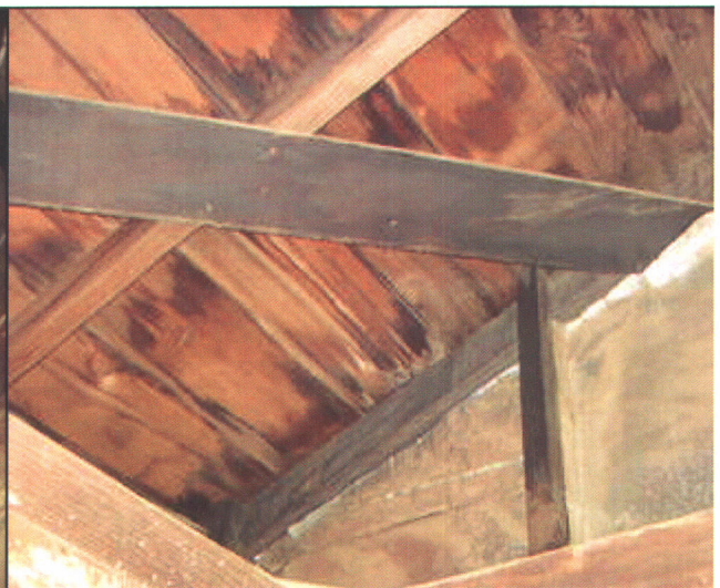
02/05/15 - Substandard Structure - NOD#11,12,13,14,17 - Pike
