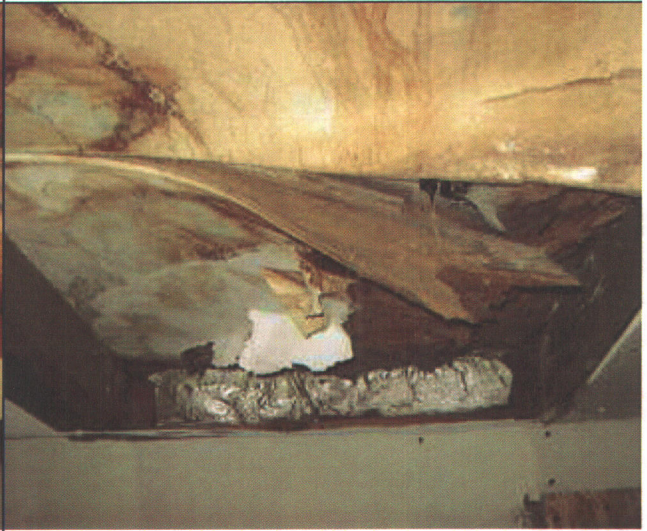
02/05/15 - Substandard Structure - NOD# 11,12,13,14,17 - Pike
