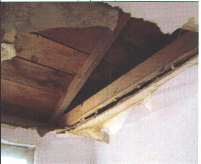
02/05/15 - Substandard Structure - NOD#11,12,13,14,17 - Pike
