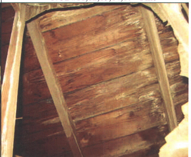
02/05/15 - Substandard Structure - NOD#11,12,13,14,17 - Pike
