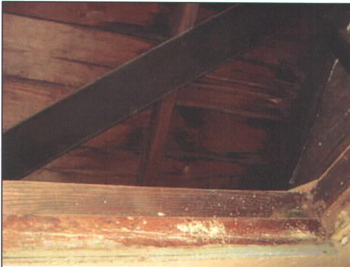
02/05/15 - Substandard Structure - NOD#11,12,13,14,17 - Pike
