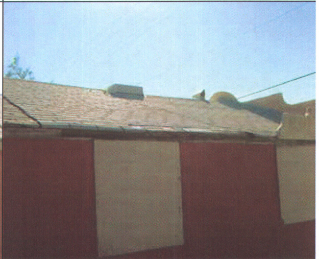
02/05/15 - Substandard Structure - NOD# 17 - P
