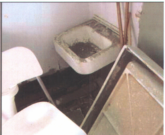
02/05/15 - Substandard Structure - NOD# 1,2,3,4,14,17 - Pike
