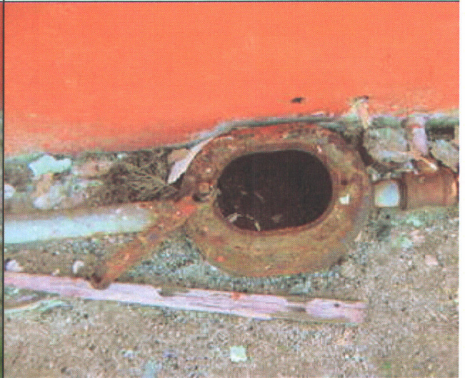
02/05/15 - Substandard Structure - NOD# 4 - Pi
