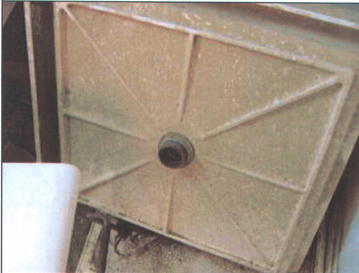
02/05/15 - Substandard Structure - NOD#1,2,3,4,14,17 - Pike
