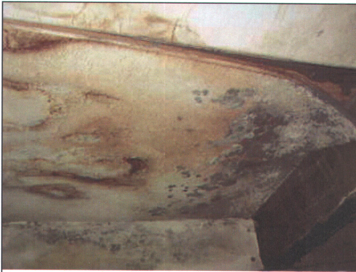
02/05/15 - Substandard Structure - NOD# 11,12,13,14,17 - Pike
