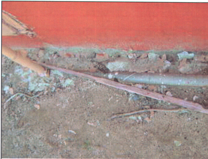
02/05/15 - Substandard Structure - NOD# 4 - Pike
