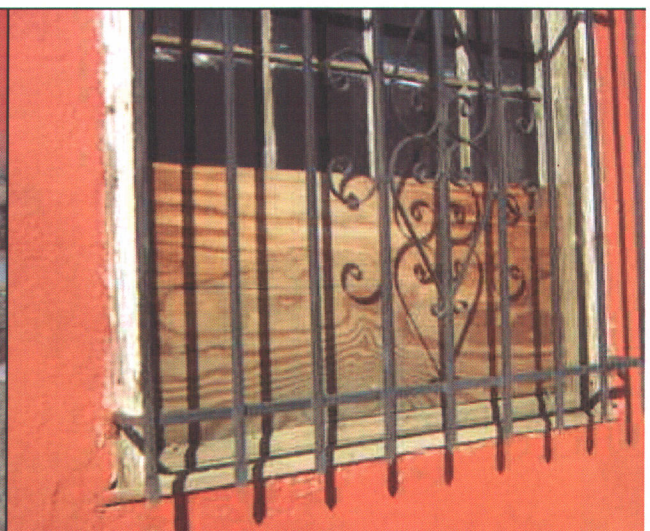
02/05/15 - Substandard Structure - NOD# 12,17 -
