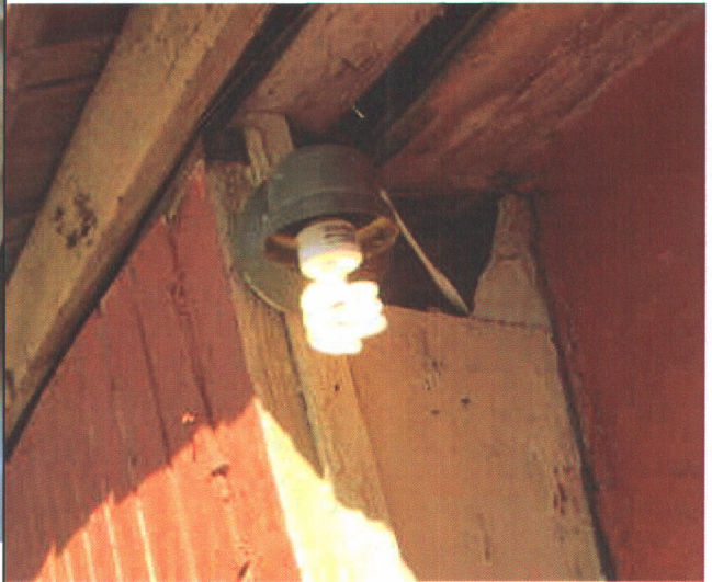
02/05/15 - Substandard Structure - NOD# 6,15 - I
