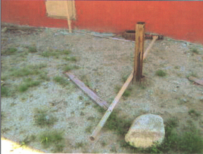
02/05/15 - Substandard Structure - NOD# 4 - Pike
