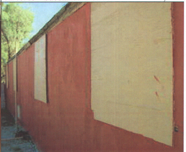
02/05/15 - Substandard Structure - NOD# 17 - P
