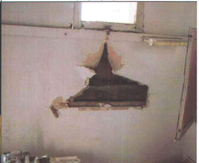
02/05/15 - Substandard Structure - NOD# 11,12,13,14,17 - Pike
