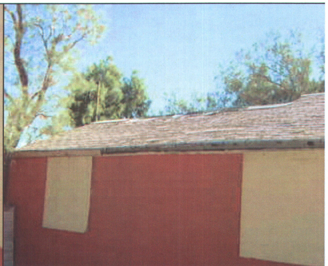
02/05/15 - Substandard Structure - NOD# - Pik
