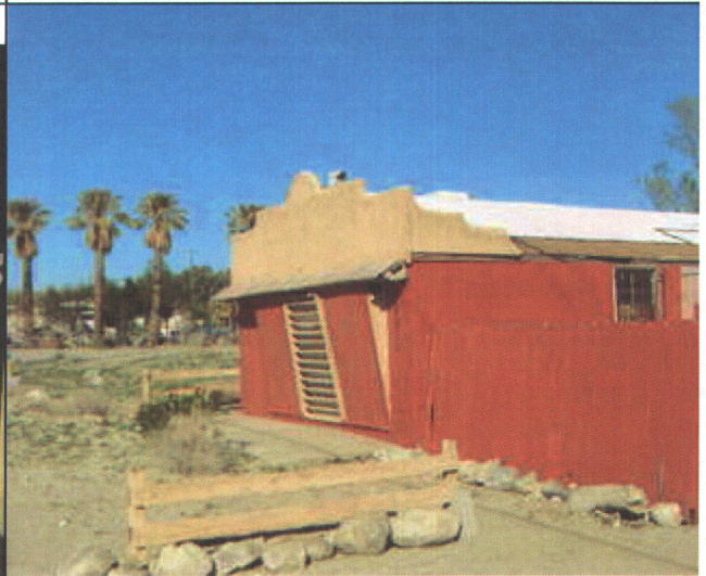
02/05/15 - Substandard Structure - NOD#11,12,13,14,17 - Pike
