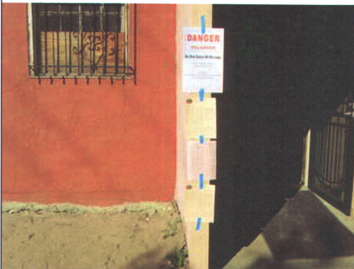
02/05/15 - Substandard Structure - Posting - Pike
