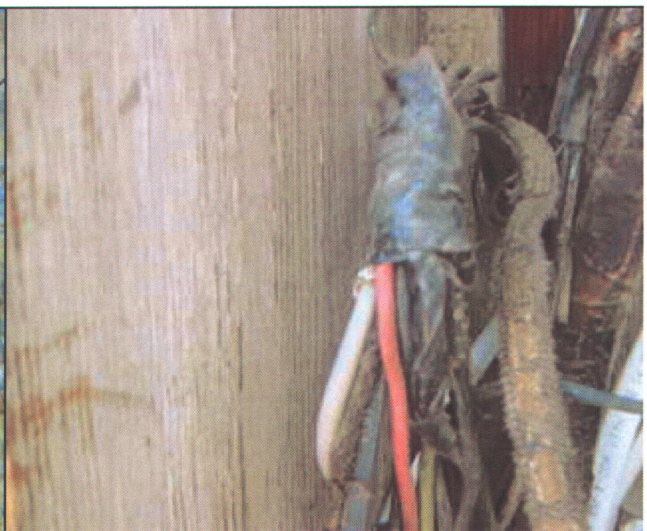
02/05/15 - Substandard Structure - NOD# 6,14,15 Pike
