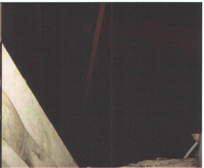
02/05/15 - Substandard Structure - NOD# 11,12,13,14,17 - Pike
