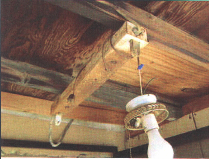
02/05/15 - Substandard Structure - NOD#6,14,15,17 - Pike
