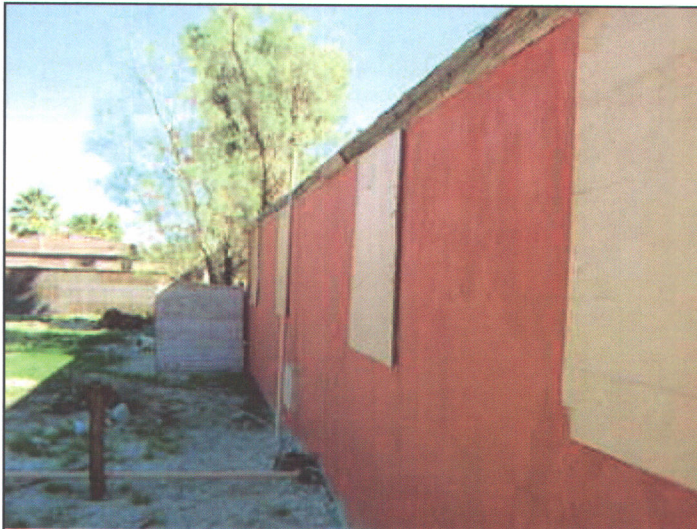
02/05/15 - Substandard Structure - NOD# 17 - Pike
