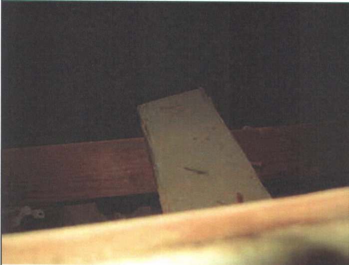
02/05/15 - Substandard Structure - NOD#11,12,13,14,17 - Pike
