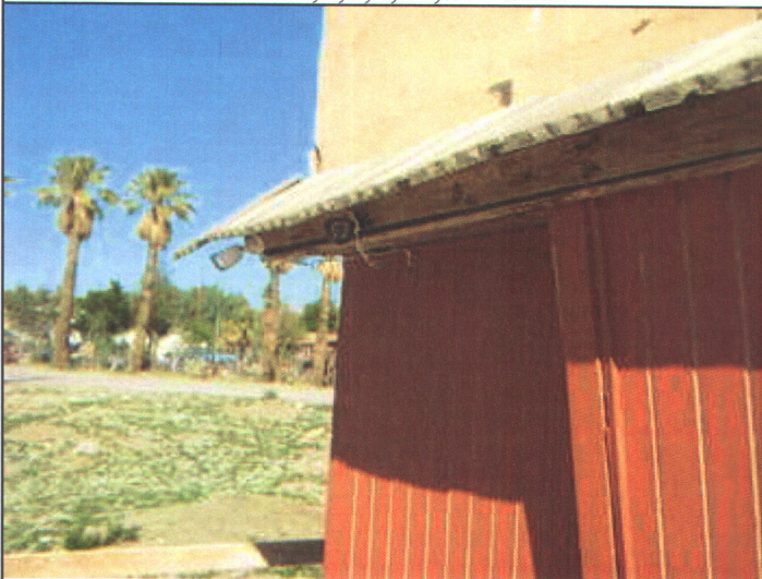
02/05/15 - Substandard Structure - NOD#17 - Pike
