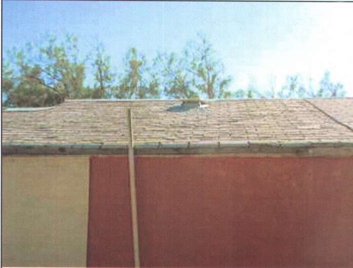
02/05/15 - Substandard Structure - NOD# 17 - Pike
