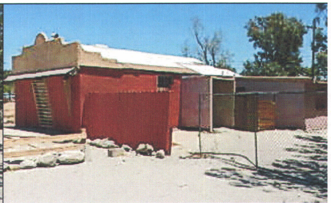
Substandard Structure 7/24/15 J. Cole
