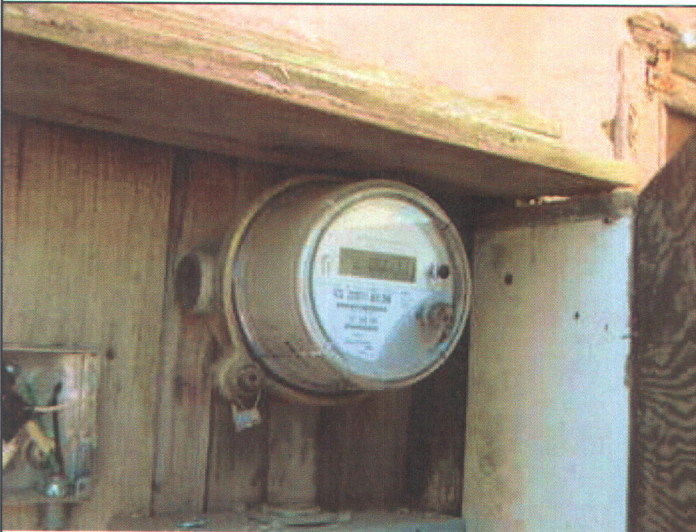
02/05/15 - Substandard Structure - NOD# 6,14,15,17 - Pike
