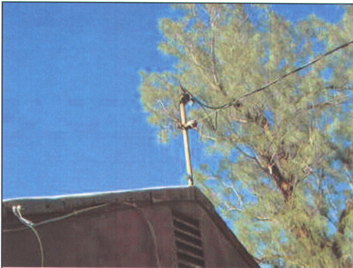
02/05/15 - Substandard Structure - NOD# 6,14,15,17 - Pike
