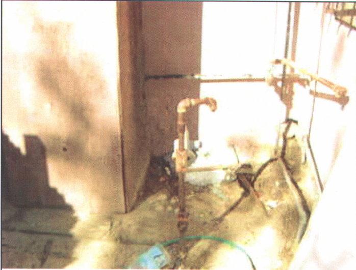
02/05/15 - Substandard Structure - NOD# 7,13,14,17 - Pike
