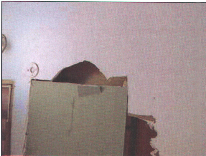
02/05/15 - Substandard Structure - NOD# 11,12,13,14,17 - Pike
