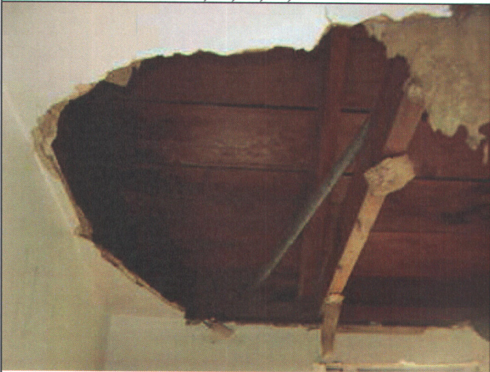
02/05/15 - Substandard Structure - NOD# 11,12,13,14,17 - Pike
