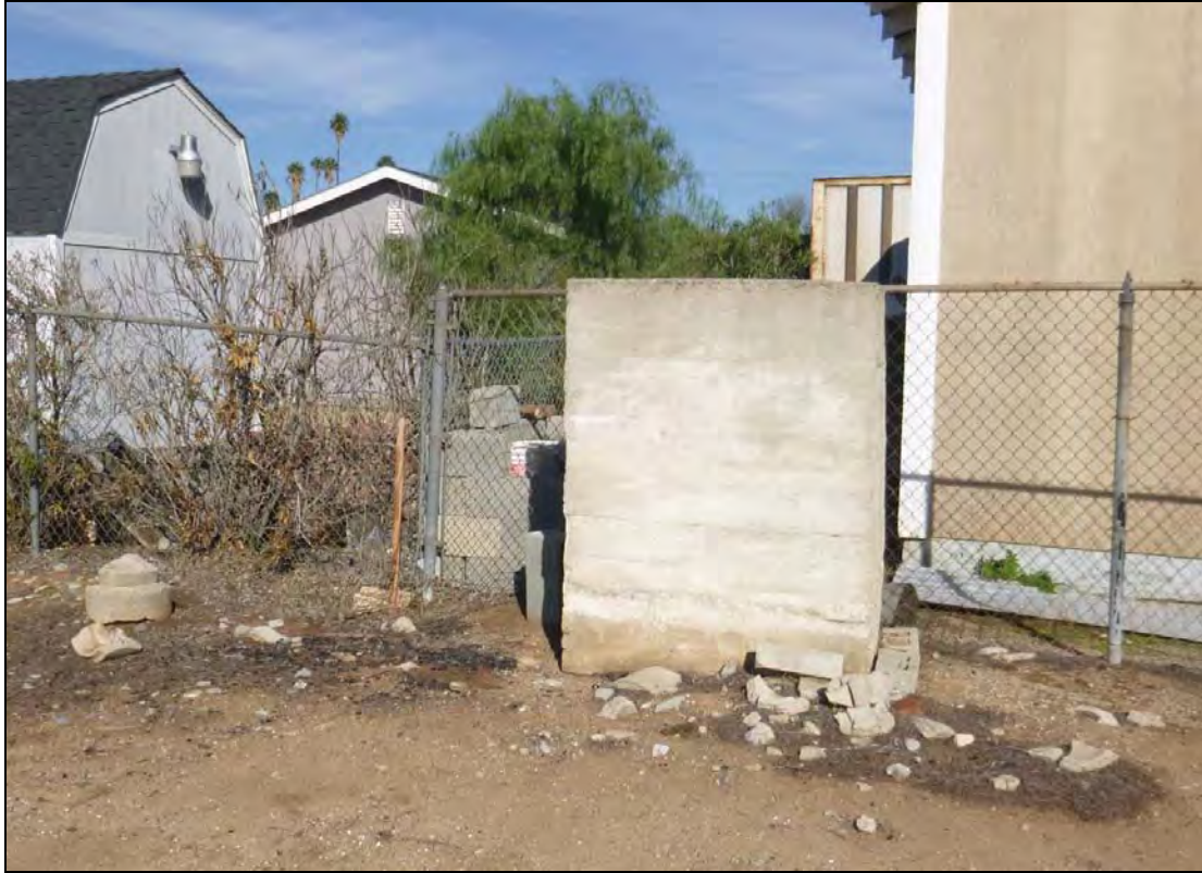
Figure 5-3 A concrete weir box (P-33-024100) next to the property fence line at the north side of the existing retention basin, view to the north.
