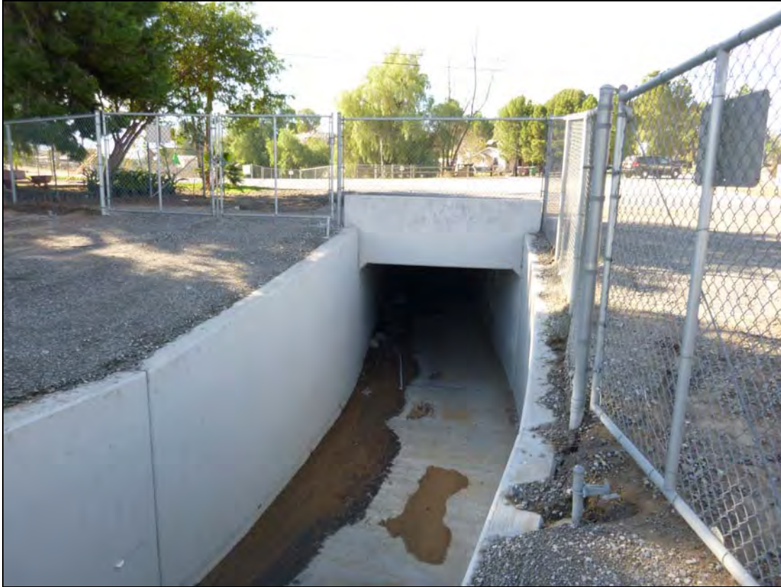
Figure 5-2 A segment of the concrete-lined open-top South Norco Channel (P-33-024099) at Corona Avenue, view to the west.
