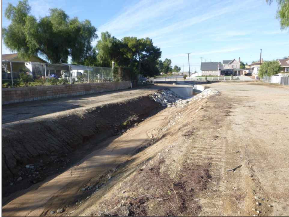
Photo 6-1 Overview of a portion of the storm channel network in the southwestern Project area, near Corona Ave., looking west.
