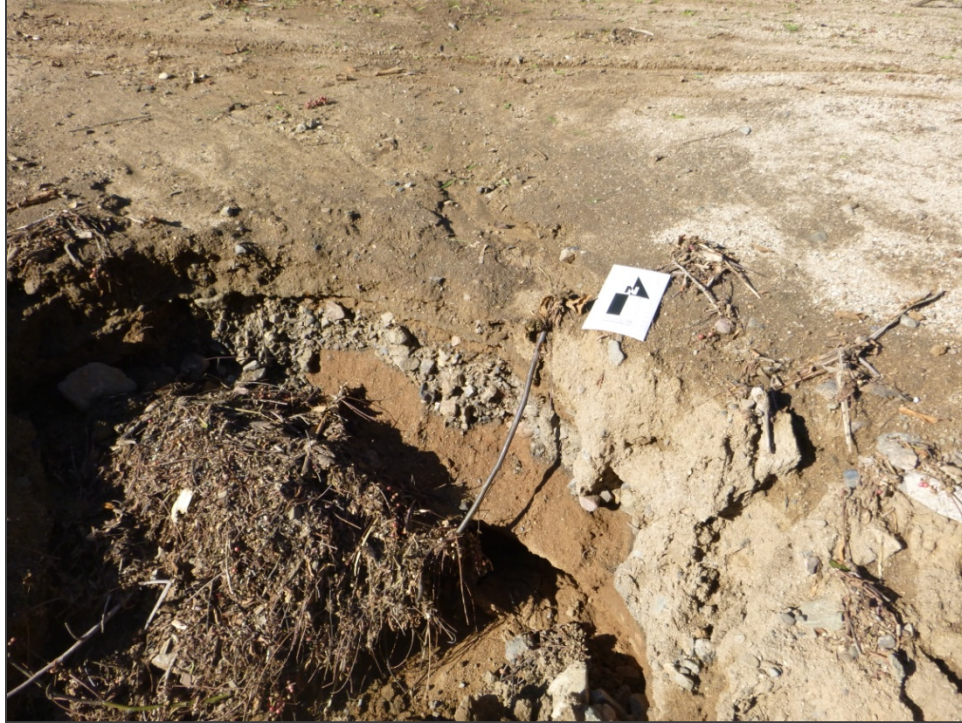
Photo 6-5 Gully erosion on the levee has exposed buried red clay soil, which is unevenly covered and truncated with imported gravel fill. View to the northeast.
