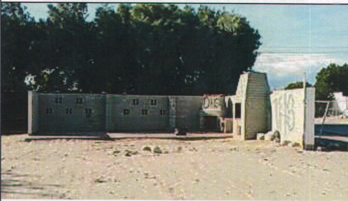
Substandard Block Wall 12/23/15 J. Cole
