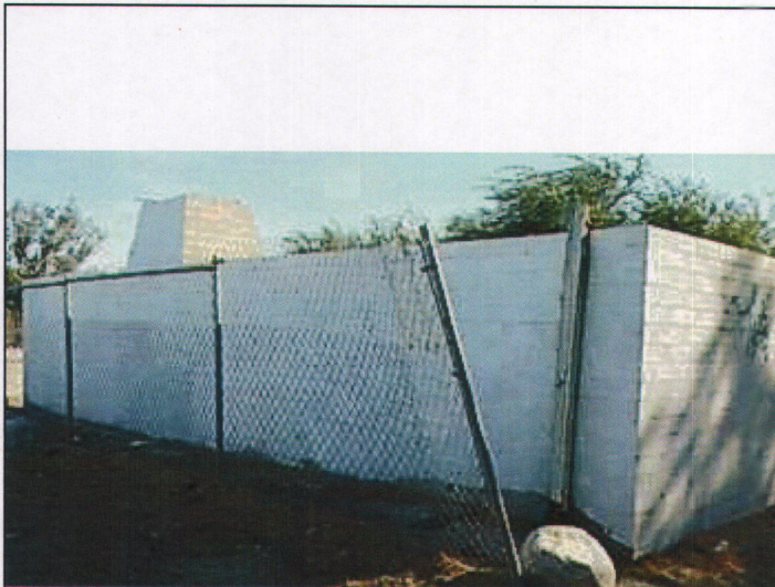
Substandard Block Wall 12/23/15 J. Cole
