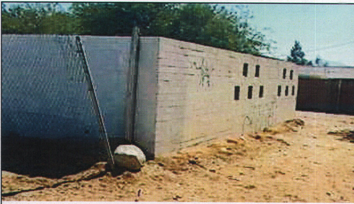
Substandard Wall 10/9/15 J. Cole
