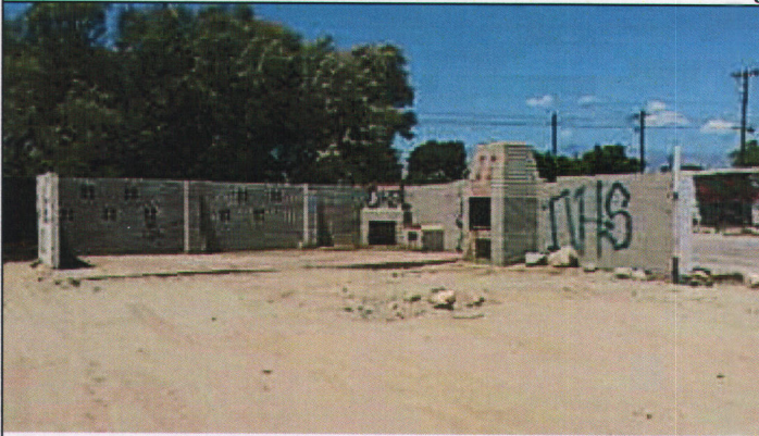
Substandard Block Wall 8/14/15 J. Cole
