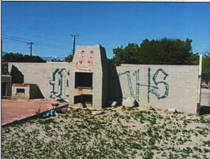
Cracks in the Wall, Graffiti 2/25/16 J. Cole
