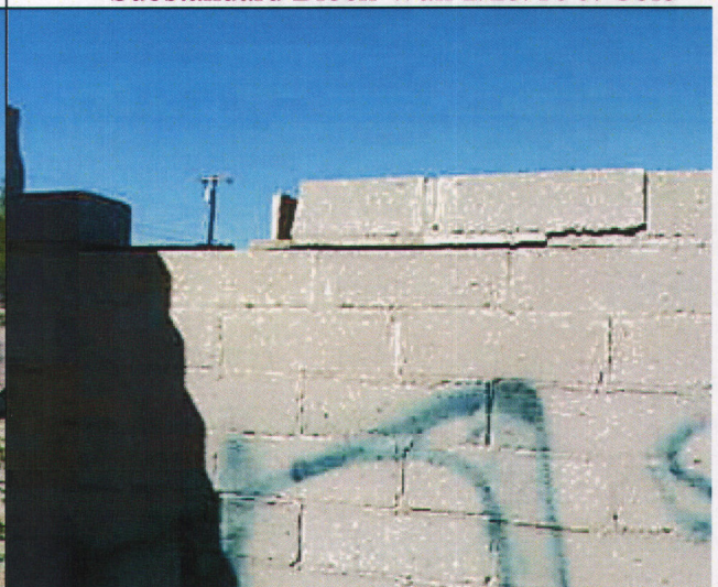
Cracks in the Wall, Graffiti 2/25/16 J. Cole
