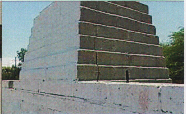
Cracks in the Block Wall 8/14/15 J. Cole
