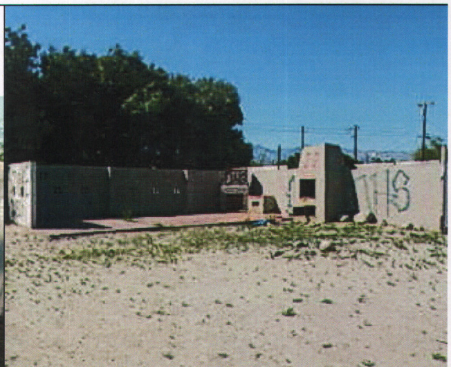
Substandard Block Wall 2/25/16 J. Cole
