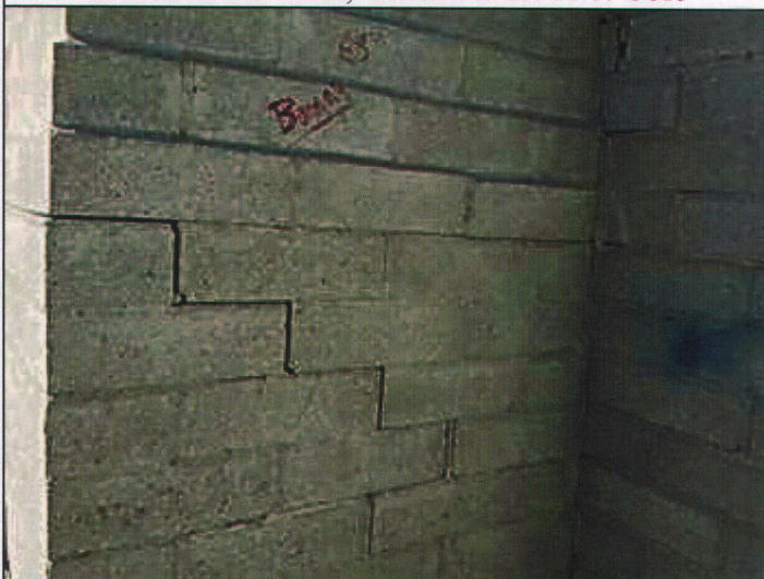
Cracks in the Wall 2/25/16 J. Cole
