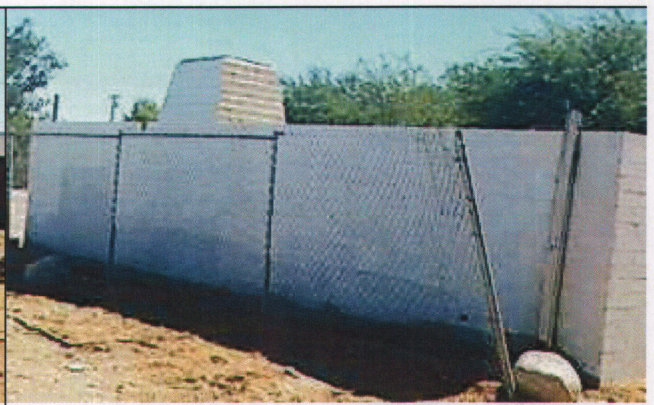
Substandard Wall 10/9/15 J. Cole
