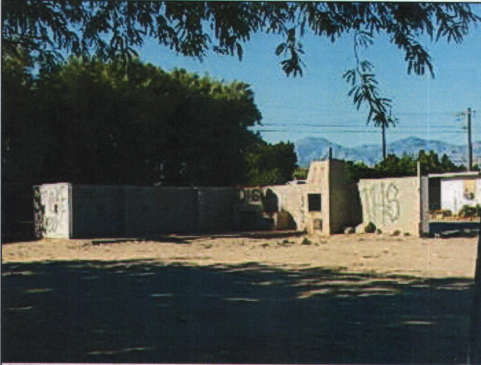
Substandard Block Wall 11/19/15 J. Cole
