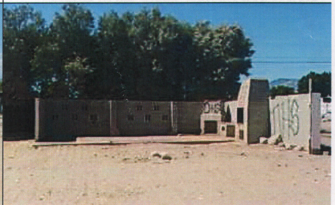
Substandard Wall 10/9/15 J. Cole
