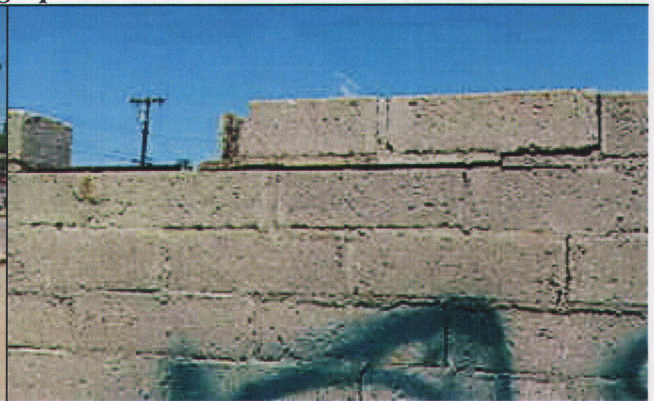
Cracks in the Block Wall 8/14/15 J. Cole
