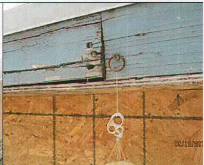
b pollard 051315 NOD's #11-Members of ceilir roofs,.....which sag, split or buckle, #13 Faulty Weather Protection, #14 General dilapidation c improper maintenance, and #18 Improper Occupa
