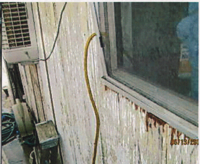
b pollard 051315 NOD's #6-Hazardous wiring, # Faulty Weather Protection, #14 General dilapidation or improper maintenance, and #18 Improper Occupancy.
