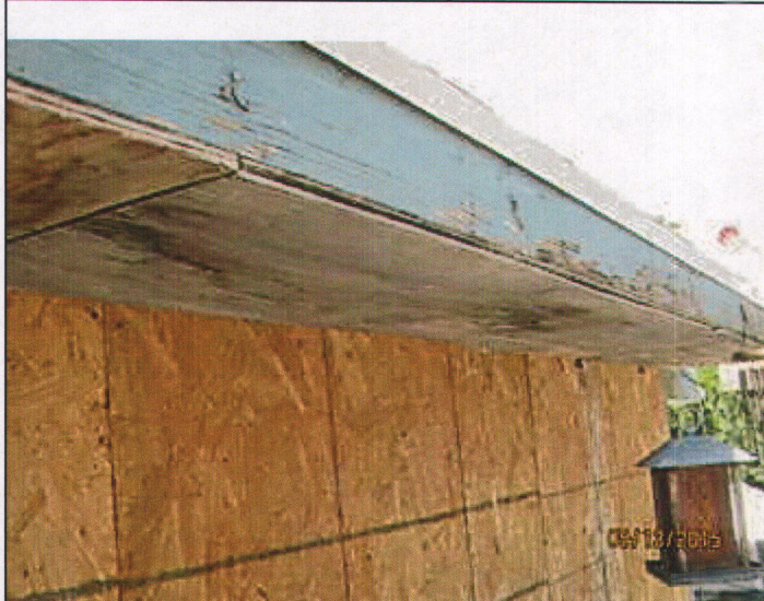
b pollard 051315 NOD's #11-Members of ceiling, roofs,.....which sag, split or buckle, #13 Faulty Weather Protection, #14 General dilapidation or improper maintenance, and #18 Improper Occupancy.
