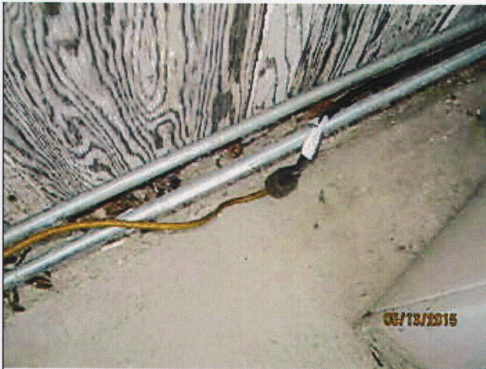
b pollard 051315 NOD's #6-Hazardous wiring, #13 Faulty Weather Protection, #14 General dilapidation or improper maintenance, and #18 Improper Occupancy.
