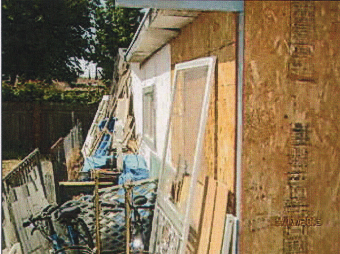
b pollard 051315 SSS, NOD's #11-Members of ceiling, roofs,.....which sag, split or buckle, #, 13 Faulty Weather Protection, #14 General dilapidation or improper maintenance, and #18 Improper Occupancy.
