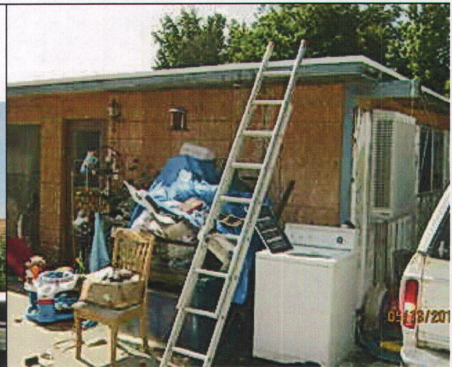
b pollard 051315 SSS-NOD #'s : #11-Members ceiling, roofs,.....which sag, split or buckle, #, 1 Faulty Weather Protection, #14 General dilapidation or improper maintenance, and #18 Improper Occupancy.
