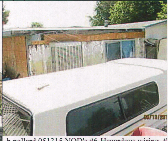
b pollard 051315 NOD's #6-Hazardous wiring, # Members of ceiling, roofs,.....which sag, split c buckle, #13 Faulty Weather Protection, #14 Gene dilapidation or improper maintenance, and #18 Improper Occupancy.
