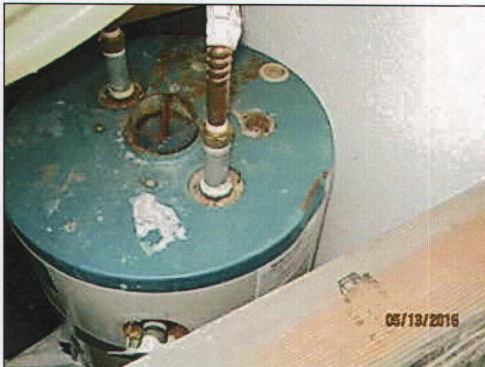
b pollard 051315 NOD's #6-Hazardous wiring, , #13 Faulty Weather Protection, #14 General dilapidation or improper maintenance, and #18 Improper Occupancy.
