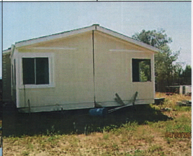
Accumulated Rubbish & Excessive Outside Storage. Lpadilla
