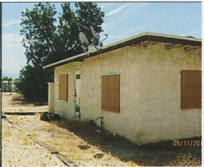
Structure now boarded up and cleaner. 1 of 8.
