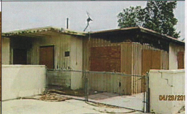
Structure remains substandard, burnt & boarded u of 6.
