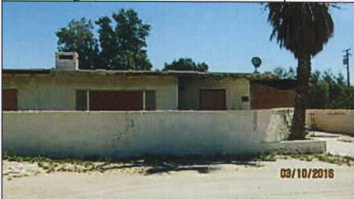
Structure remains substandard, burnt, boarded up and free of trash. 1 of 8.
