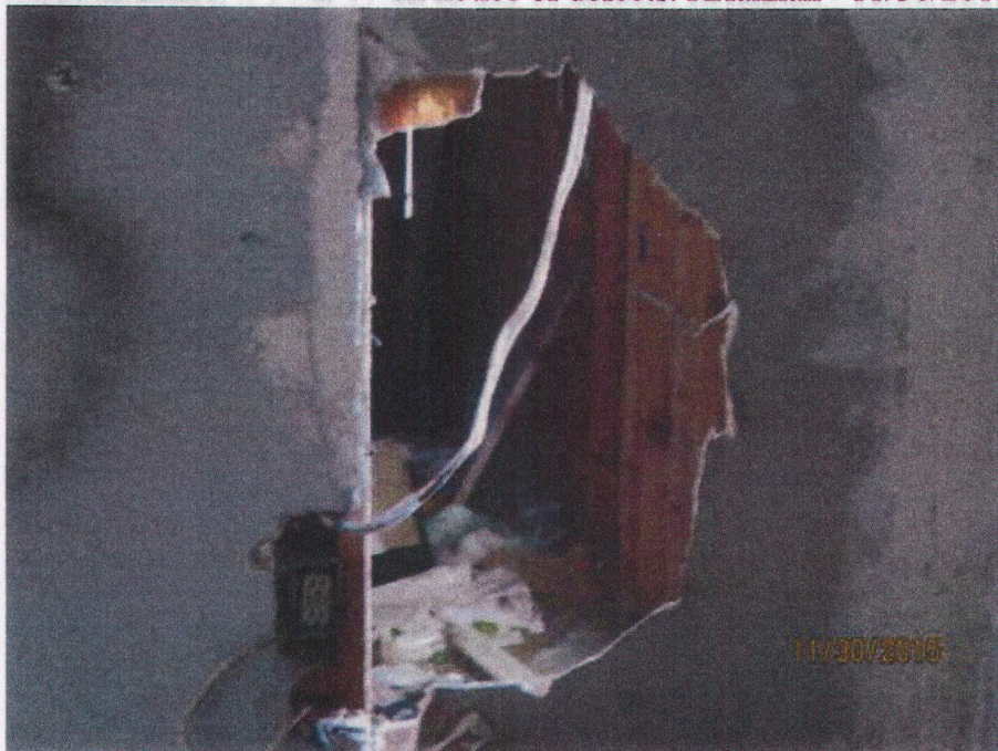
Inside structure. # 14 & 17 on notice of defects. RHannah - 11/30/2015
