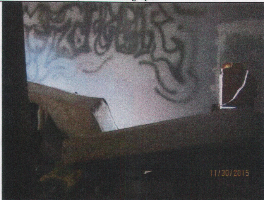
Inside structure. # 14 & 17 on notice of defects. RHannah - 11/30/2015
