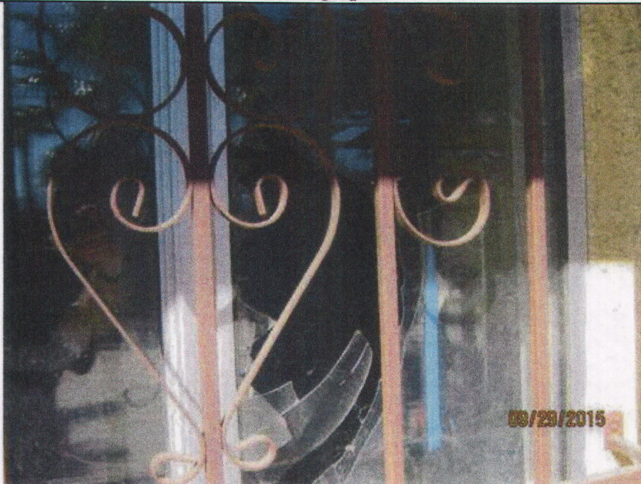
Broken window*, # 14 & 17 on notice of defects. RHannah - 09/29/2015
