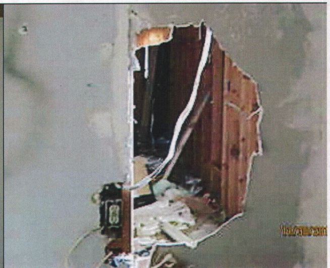
Inside structure. # 14 & 17 on notice of defects RHannah
