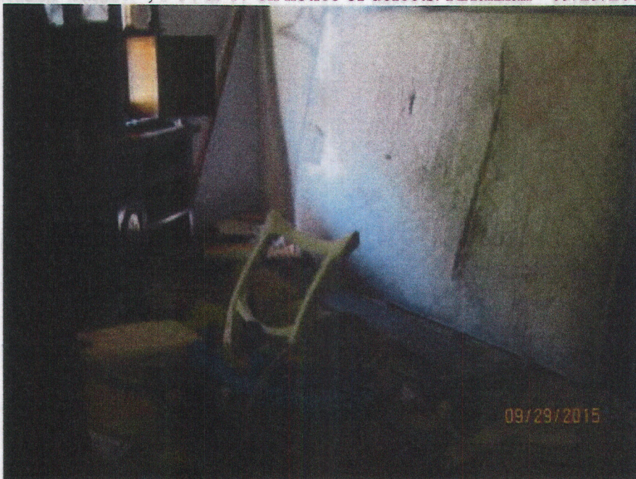
Inside structure*. # 14 & 17 on notice of defects. RHannah - 09/29/2015
