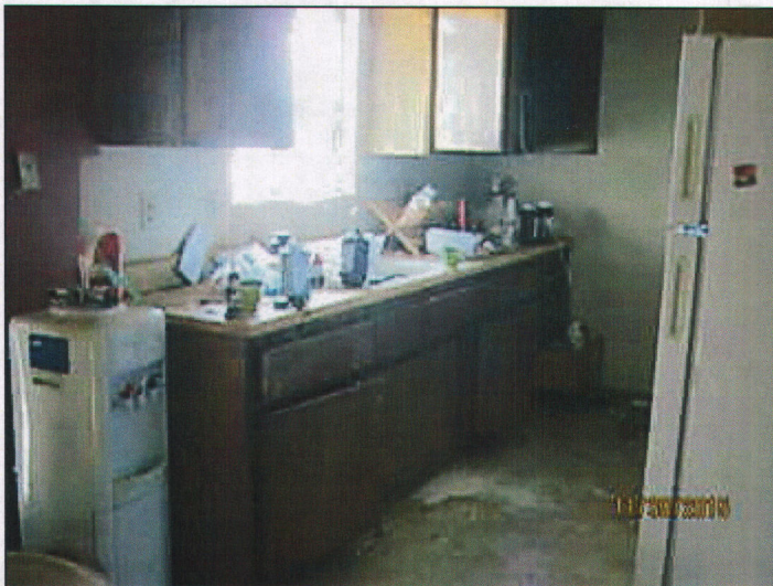
Inside structure'. # 14 & 17 on notice of defects. RHannah
