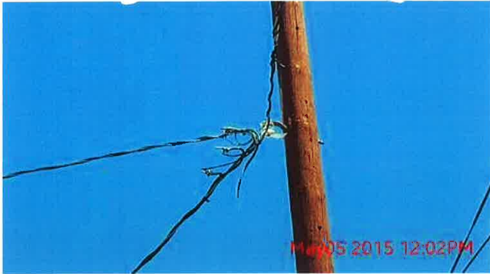
E. Torres; SS 1&2- defects 5 - 05/05/2015
