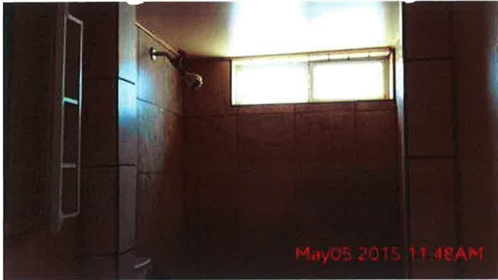
E. Torres; SS2- defects 1, 2, 4, 17, 19 - 05/05/2015
