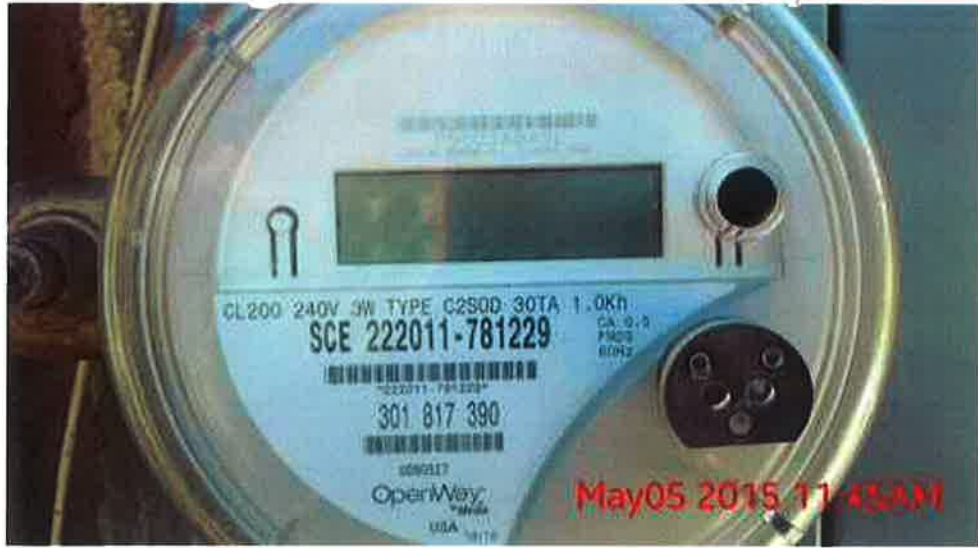
E. Torres; electric meter - 05/05/2015
