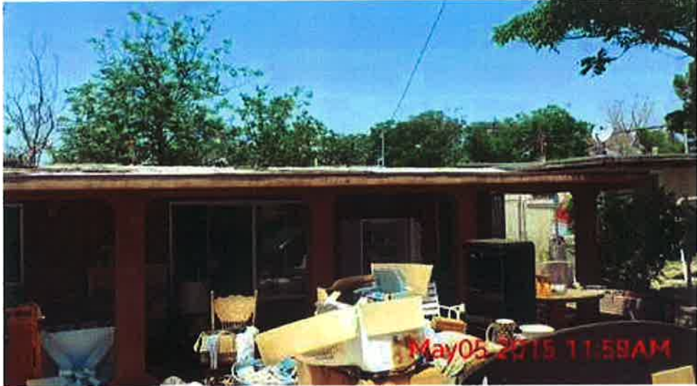
E. Torres; SS1- defects 14, 17, 19 - 05/05/2015
