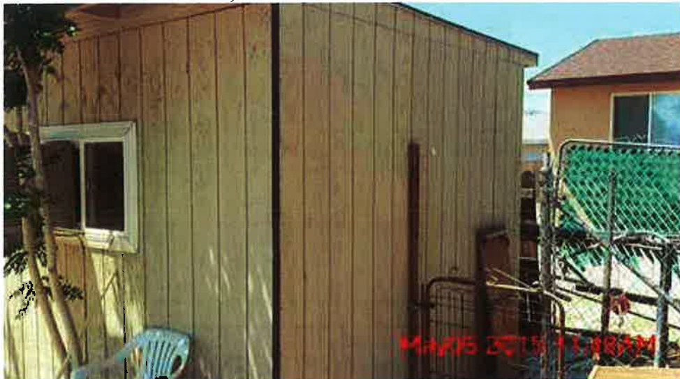
E. Torres; SS2- defects 13, 14, 17, 19 - 05/05/2015
