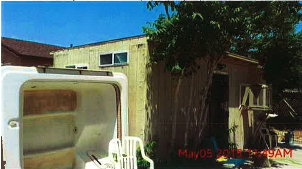
E. Torres; SS2- defects 10, 13, 14, 17, 19 - 05/05/2015
