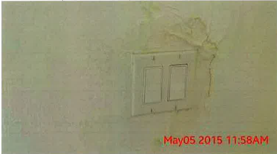
E. Torres; SS1- defects 6, 12, 13, 14, 17, 19 - 05/05/2015
