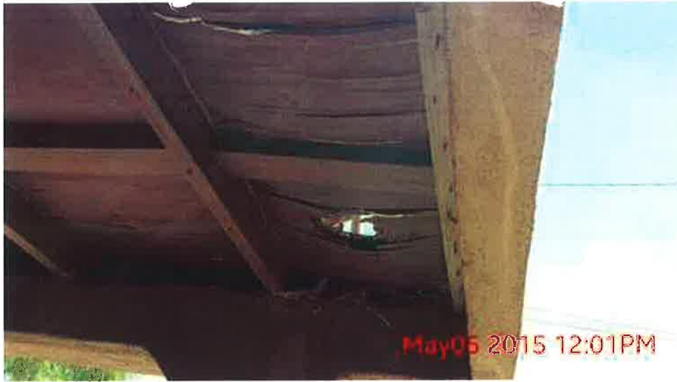
E. Torres; SS1- defects 11, 13, 14, 17, 19 - 05/05/2015
