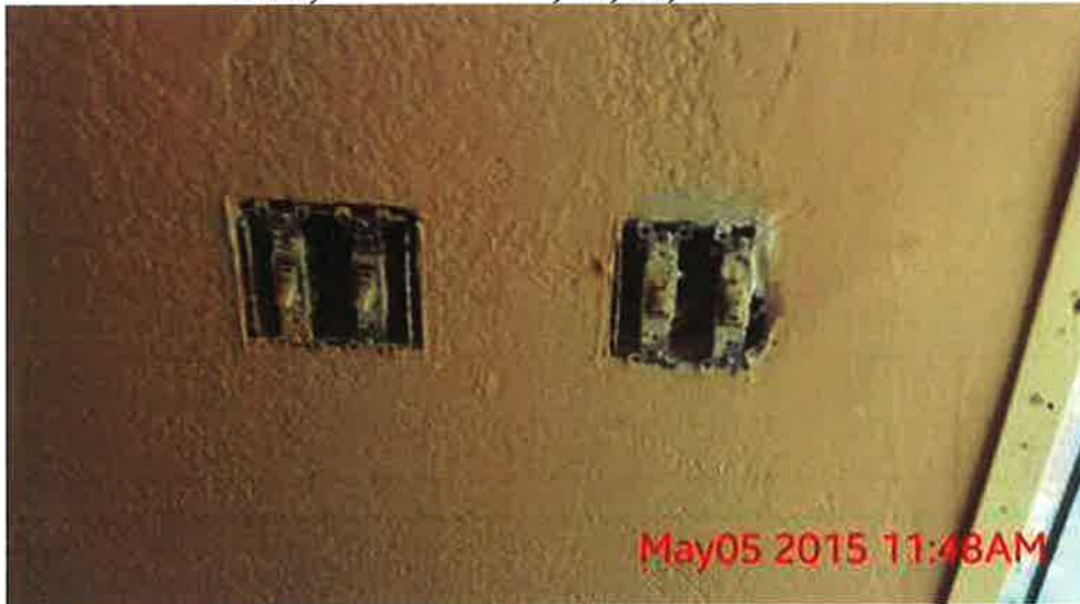
E. Torres; SS2- defects 6, 14, 17, 19 - 05/05/2015
