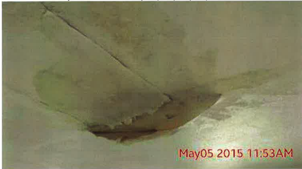
E. Torres; SS1- defects 11, 12, 13, 14, 17, 19 - 05/05/2015
