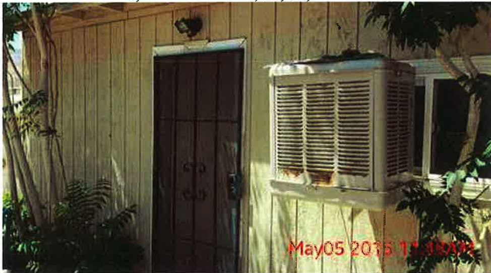
E. Torres; SS2- defects 13, 14, 17, 19 - 05/05/2015
