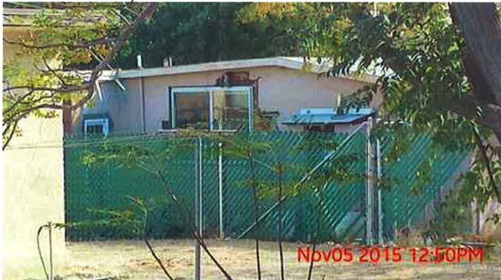
E. Torres; substandard structure with broken stucco - 11/05/2015
