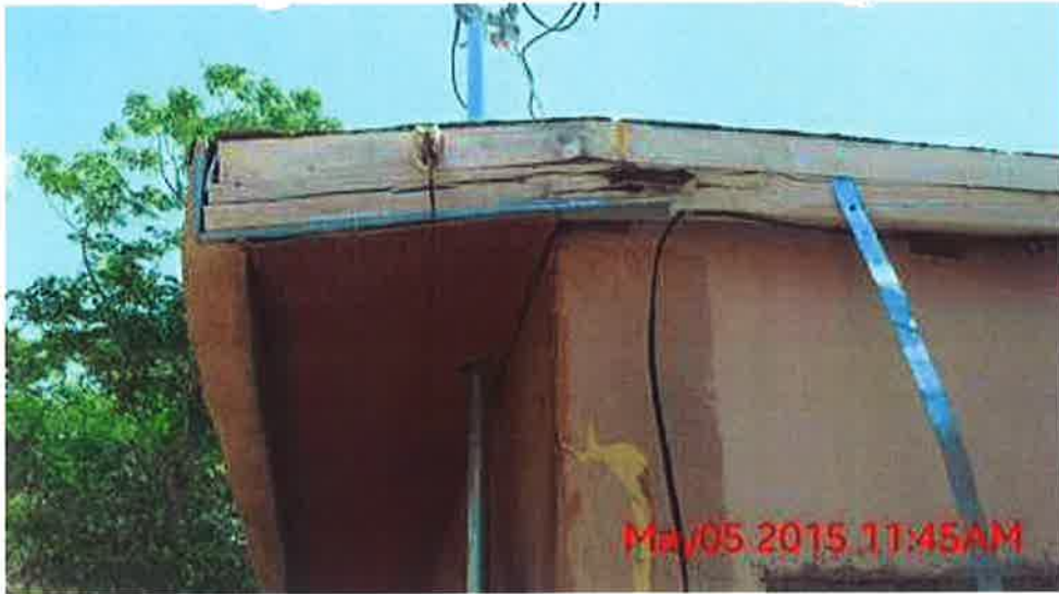
E. Torres; SS1- defects 11, 13, 14, 17, 19 - 05/05/2015
