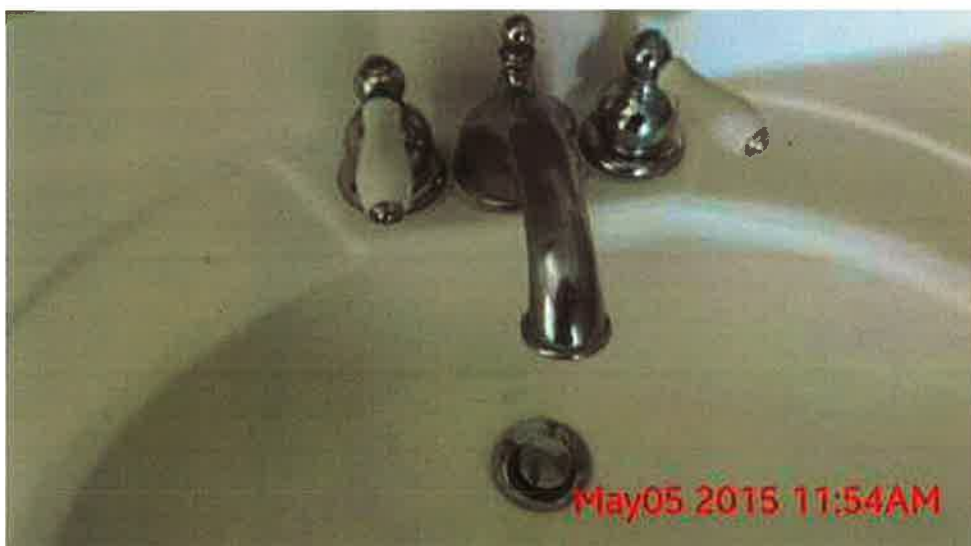
E. Torres; SS1- defects 1, 2, 14, 17 - 05/05/2015
