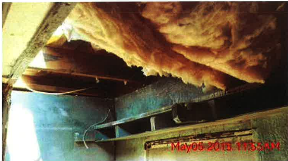
E. Torres; SS1- defects 11, 12, 13, 14, 17, 19 - 05/05/2015
