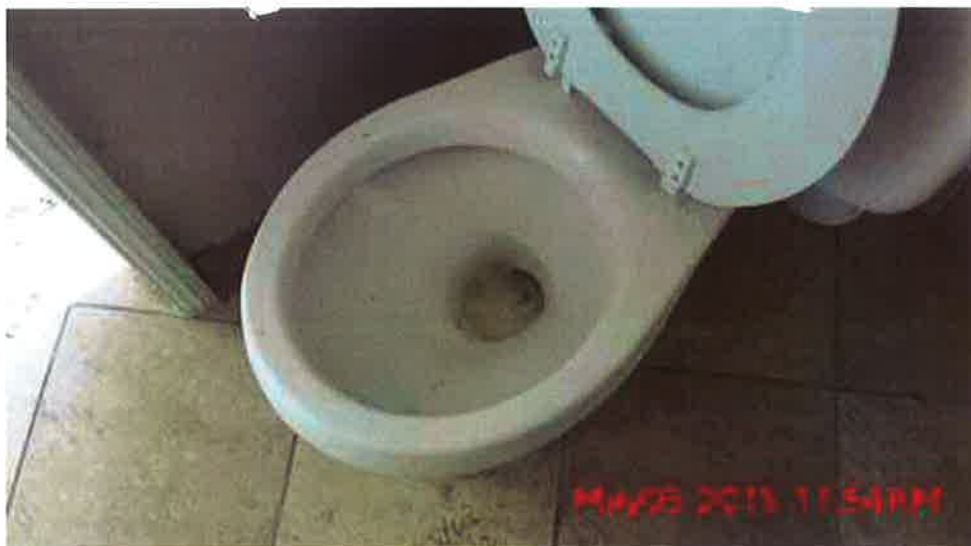
E. Torres; SS1- defects 1, 2, 14, 17 - 05/05/2015
