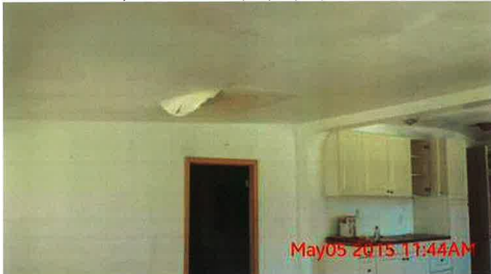
E. Torres; SS1- defects 11, 12, 13, 14, 17, 19 - 05/05/2015
