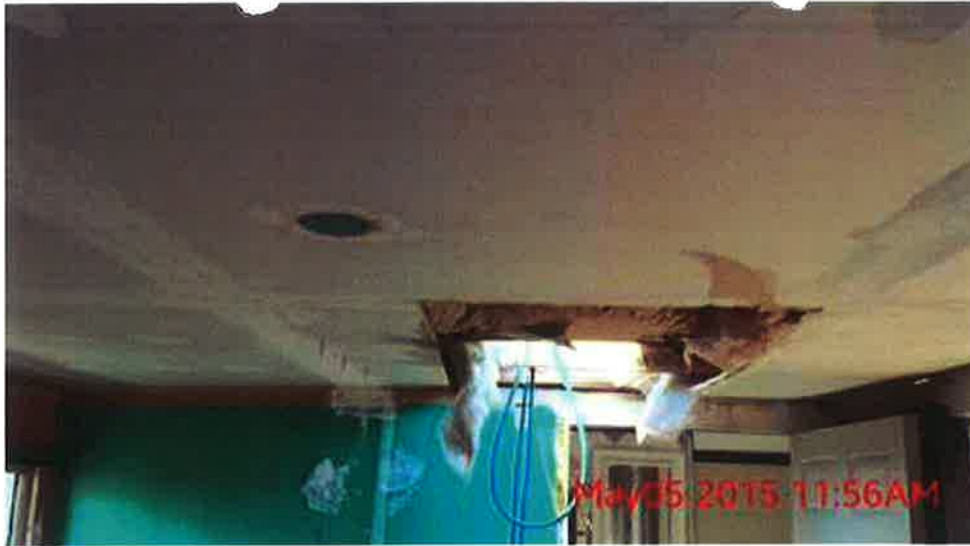
E. Torres; SS1- defects 11, 12, 13, 14, 17, 19 - 05/05/2015
