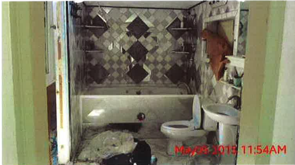
E. Torres; SS1- defects 13, 14, 17, 19 - 05/05/2015
