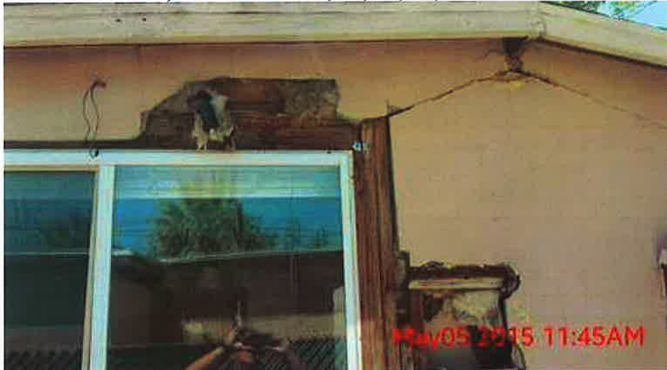
E. Torres; SS1- defects 10, 13, 14, 17, 19 - 05/05/2015
