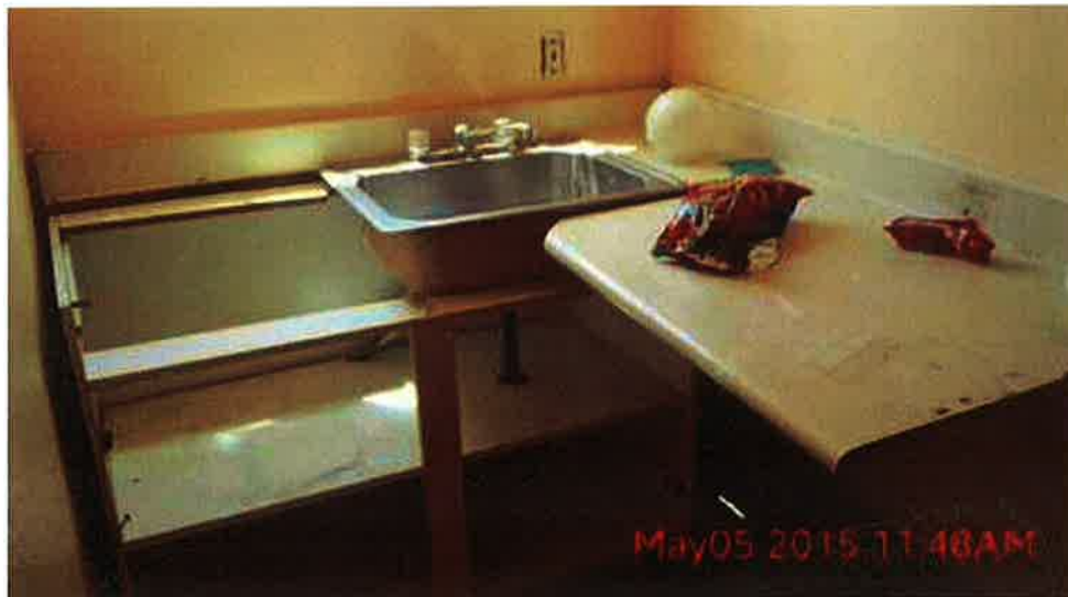
E. Torres; SS2- defects 1, 2, 4, 17, 19 - 05/05/2015
