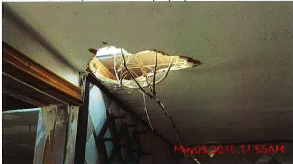
E. Torres; SS1- defects 11, 12, 13, 14, 17, 19 - 05/05/2015
