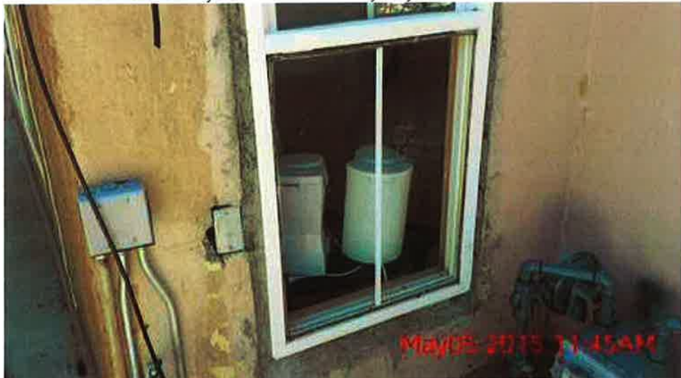
E. Torres; SS1- defects 10, 13, 14, 17, 19 - 05/05/2015
