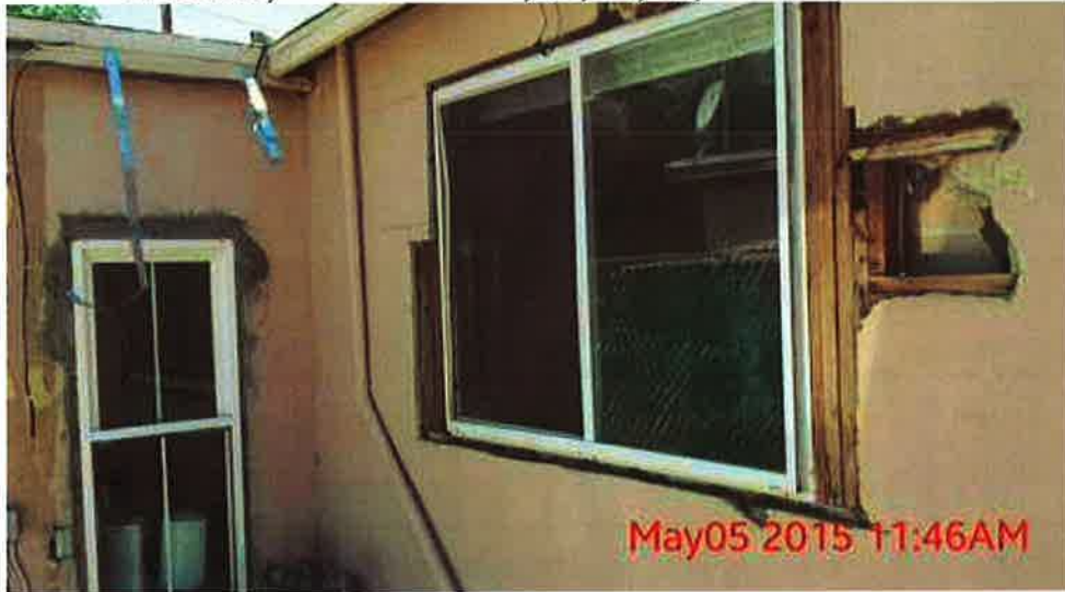
E. Torres; SS1- defects 10, 13, 14, 17, 19 - 05/05/2015
