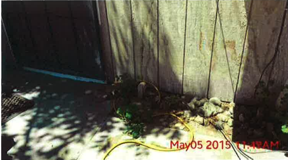
E. Torres; SS2- defects 5, 6, 13, 14, 17, 19 - 05/05/2015
