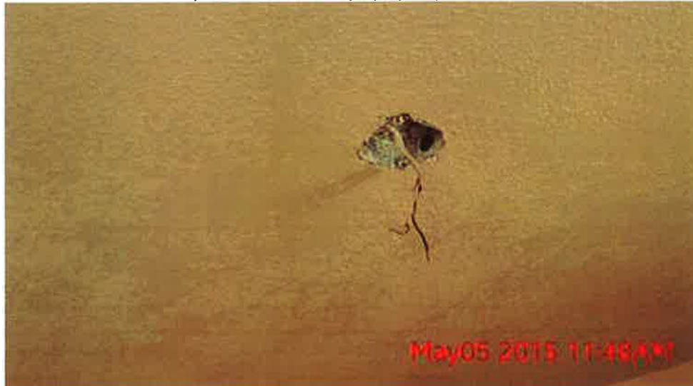
E. Torres; SS2- defects 5, 6, 11, 15, 17, 19 - 05/05/2015
