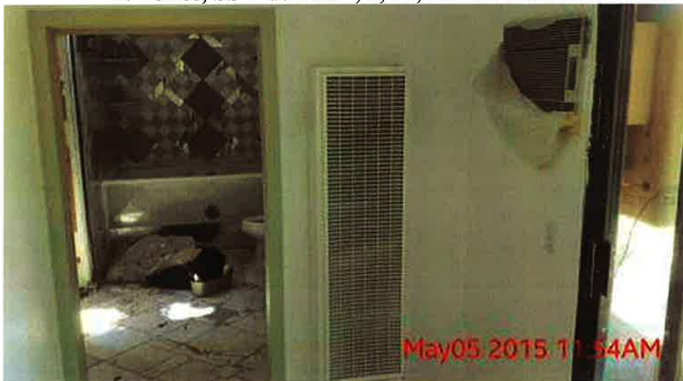
E. Torres; SS1- defects 13, 14, 17, 19 - 05/05/2015
