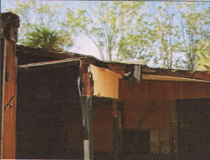
110215 TM missing roof section
