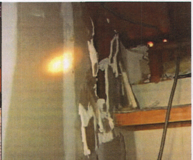
110215 TM damaged drywall
