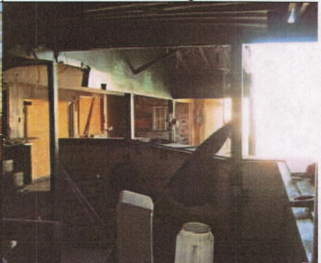
110215 TM missing wall and roof
