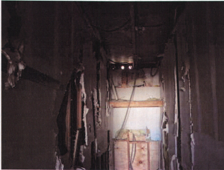
110215 TM damaged interiors - 11/03/2015
