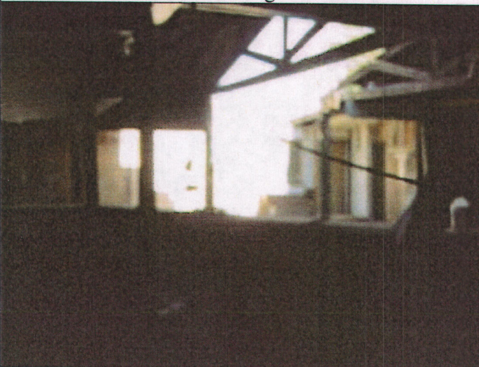
110215 TM missing wall and roof
