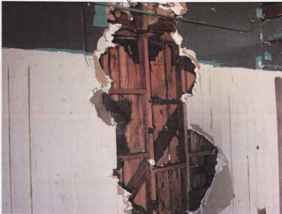
110215 TM damaged exterior wall - 11/03/2015
