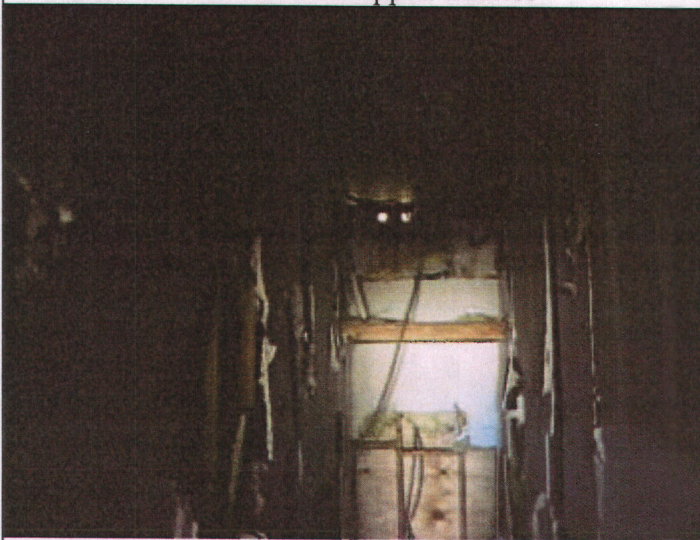
110215 TM damaged interiors
