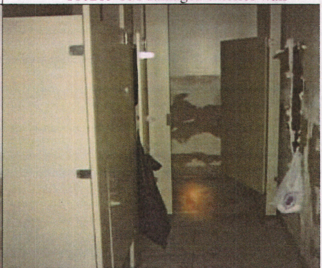
110215 TM damaged bathroom
