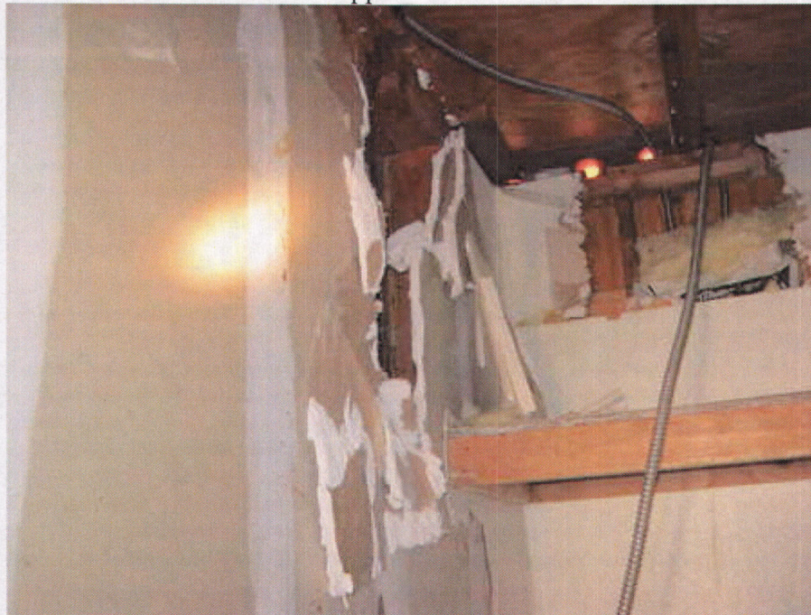
110215 TM damaged drywall - 11/03/2015
