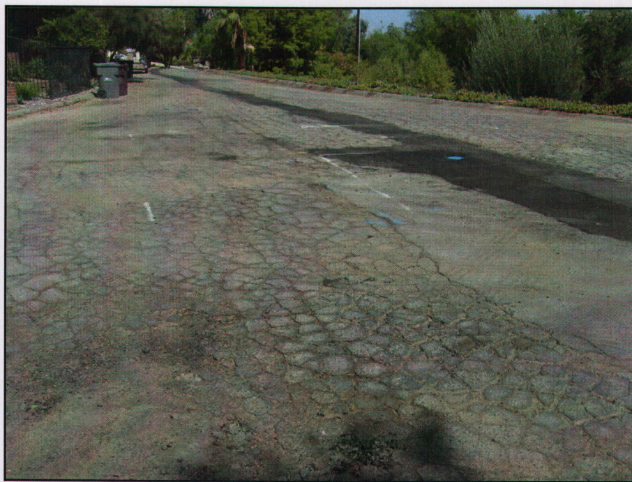
Figure 11F. PCI<10 (Very Poor Condition)
