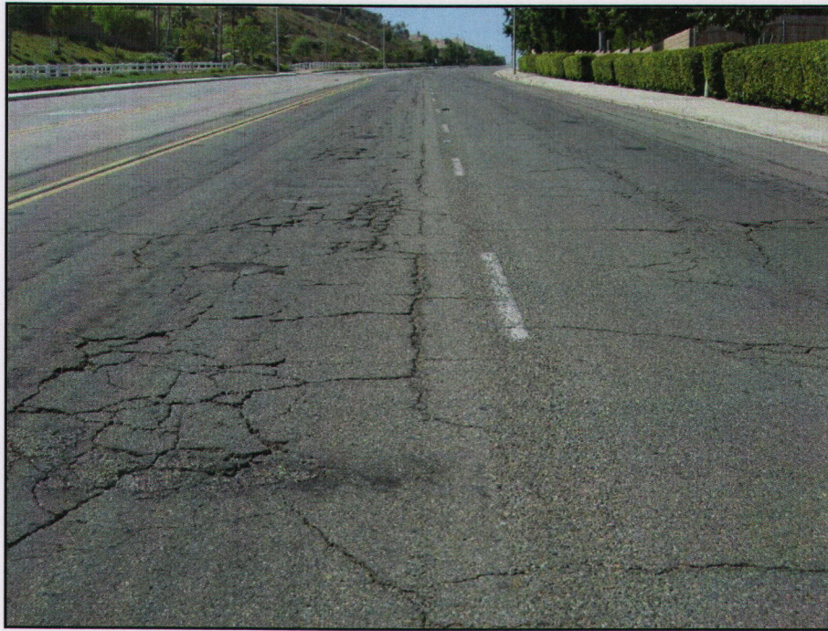
Figure 11E. PCI=30 (Poor Condition)
