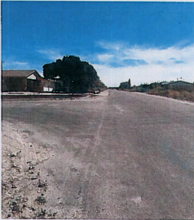
North Shore — Salton View Drive and Via Costa Brava intersection: Lacks yield or stop signs, lighting, crosswalks, or road markings.
