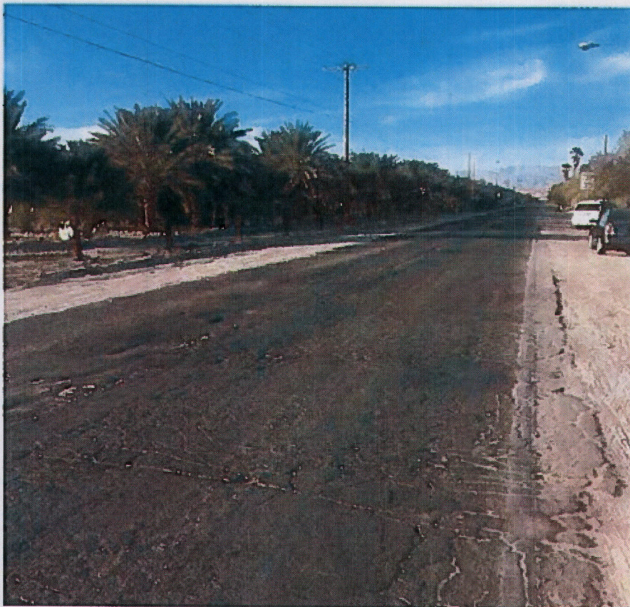
Mecca — Lincoln Street: poorly paved road in need of repair. Potholes cause cars to swerve causing danger to pedestrians and other motorists.
