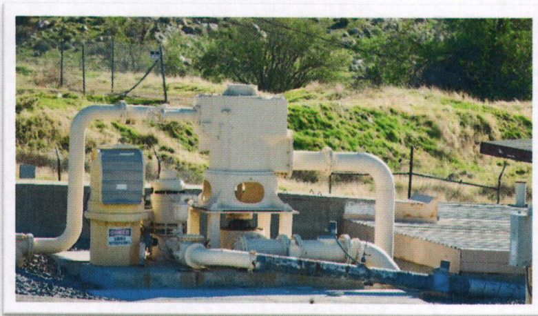
City of Banning production well located in the San Gorgonio River Valley
