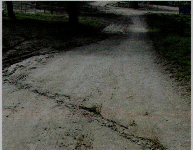
Erosion/drainage issues along the dirt roads.
