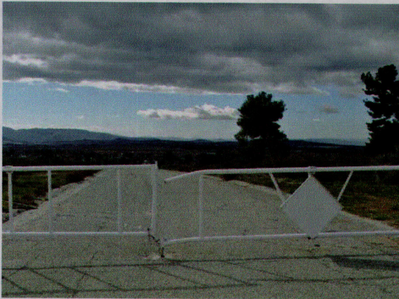
Vehicular gate in need of repair.
