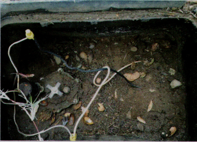
Sediment filled irrigation control box.
