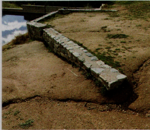
Stone wall eroding with soil in need of repair or replacement.
