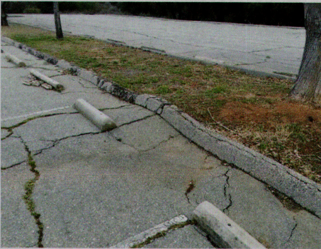
Example of the damage done to asphalt parking lot/curbs from adjacent trees, this will need to be rebuilt.
