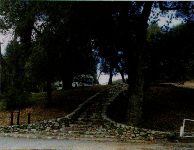
Cobble stairs in good condition, but sediment/erosion issues on the road below.
