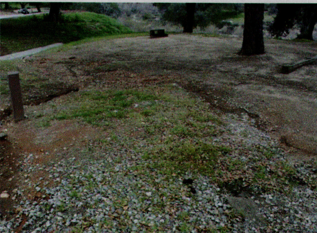
Erosion/drainage issues along the dirt roads.
