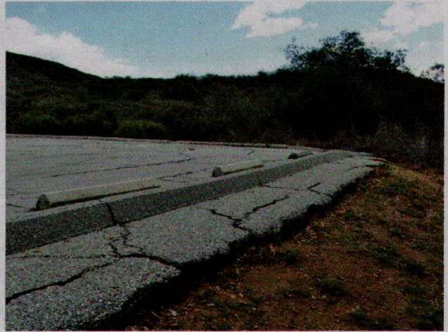
Erosion surrounding a parking lot in need of repair.
