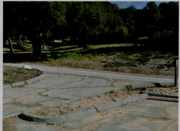
Example of the pavement and curb with erosion control repairs that are required.
