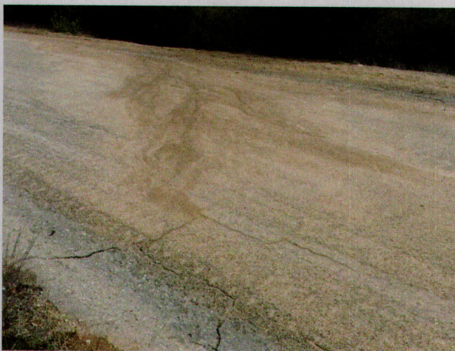
Light erosion and sediment deposition on a roadway.
