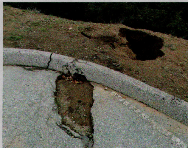
Severe erosion conditions on the edge of a parking lot/curb.
