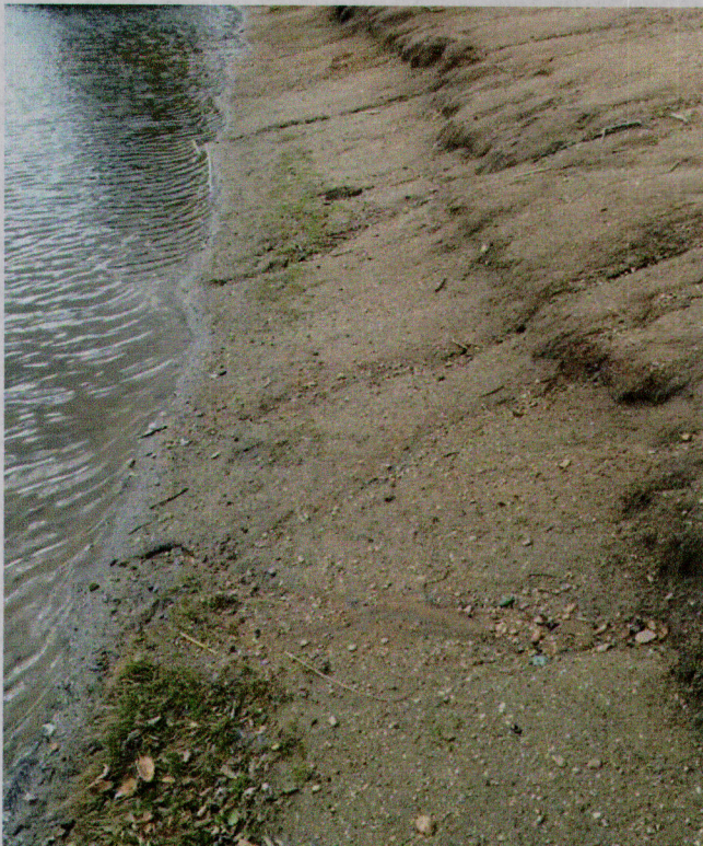
Erosion into the pond.
