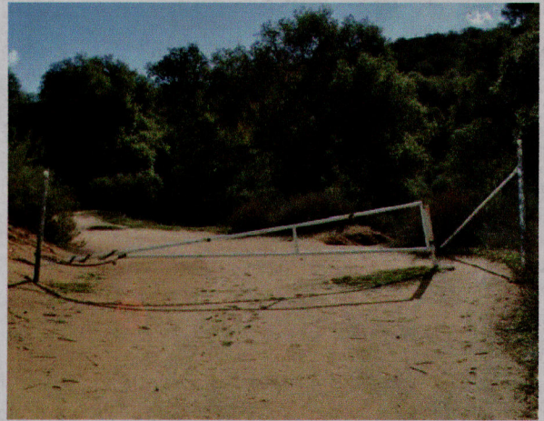
Access gate in need of repair.
