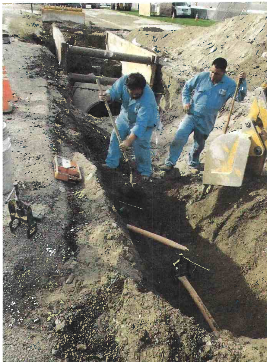
Photo 1 - Gas Line Discovered in Storm Drain Alignment
