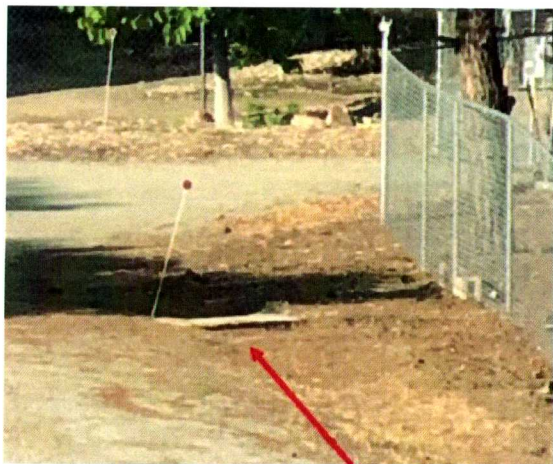
Applicant's non-permitted drainage pop-up system in part of Cibola Circle
