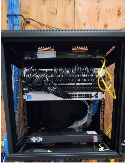
Figure 3 Patch Panels in Cabinet
