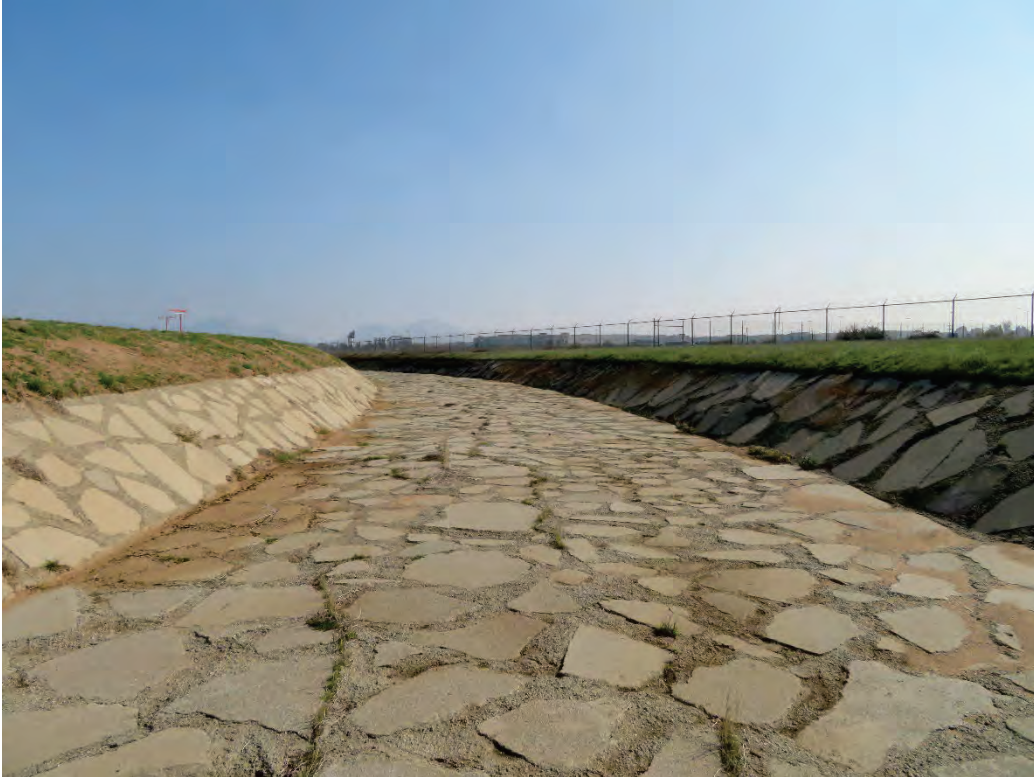
Photograph 7: View of concrete-lined portion of the PVC (South Segment) in the southern portion of the project site, facing east (downstream).
