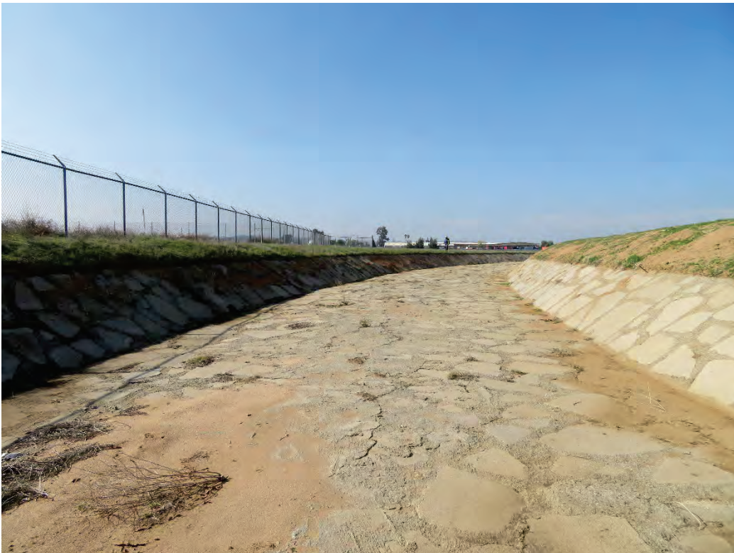
Photograph 8: View of concrete-lined portion of the PVC (South Segment) in the southern portion of the project site, facing west (upstream).
