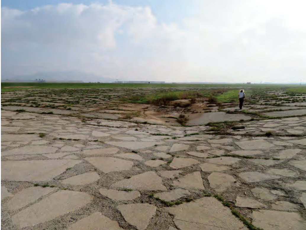
Photograph 3: View of concrete-lined portion of the PVC (North Segment) in the northern portion of the project site, facing southeast (downstream).
