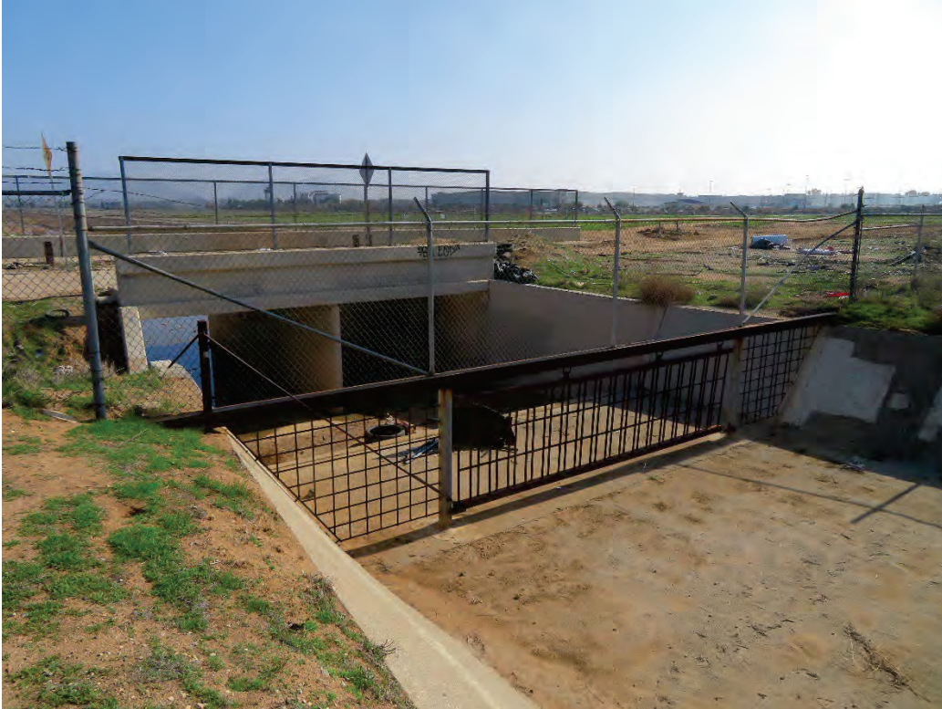
Photograph 9: View of Heacock Street crossing over the PVC (South Segment) in the southeast corner of the project site, facing southeast (downstream).
