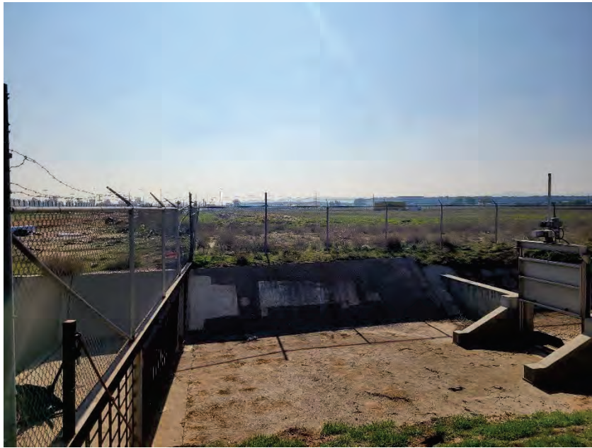
11. View of flood control equipment in southern portion of Site
