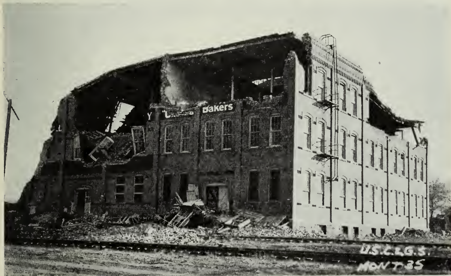
FIG. 1. What happened to a building not designed to resist earthquakes. Helena, Montana, 1935.
