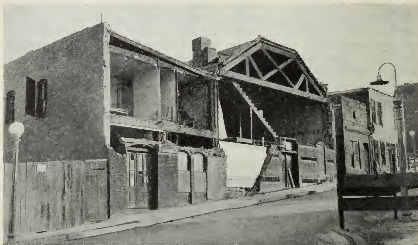
FIG. 2. The front of this building was shaken down by the Helena, Montana, earthquake of 1935.
