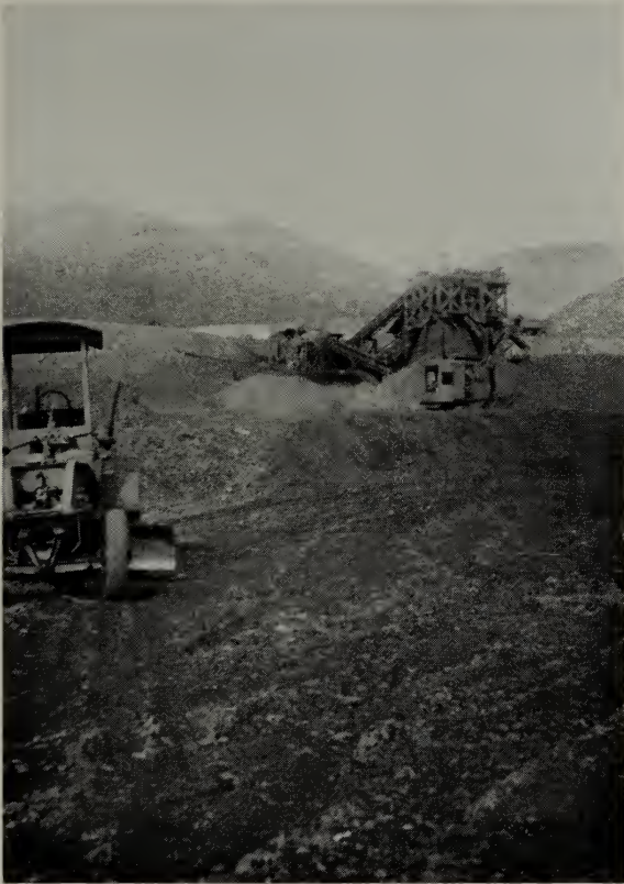
CRUSHING AND SCREENING PLANT OF MINERAL MATERIALS COMPANY ON EAGLE MOUNTAINS IRON DEPOSIT, RIVERSIDE COUNTY
