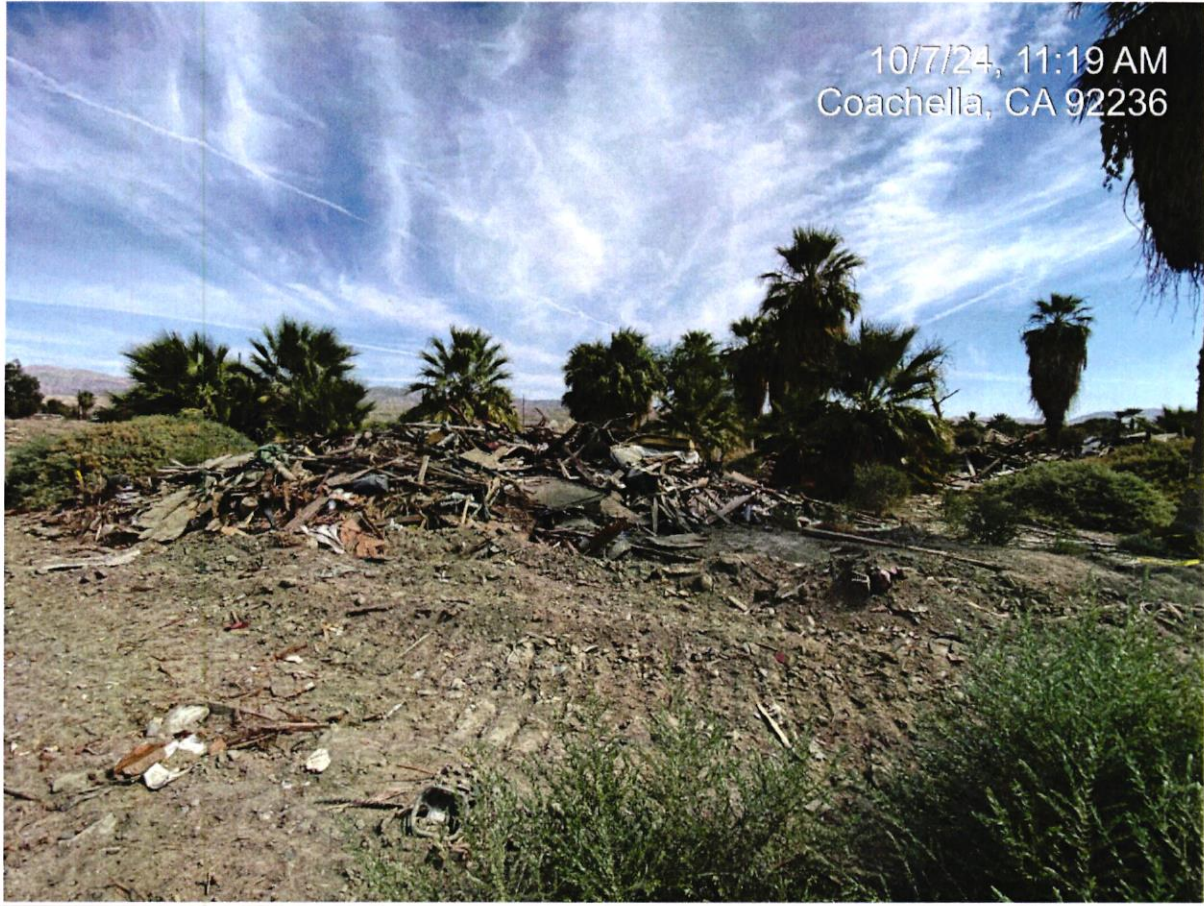
Debris field/demolished structure with positive Asbestos, northeast viewpoint of east side area of Section E.
