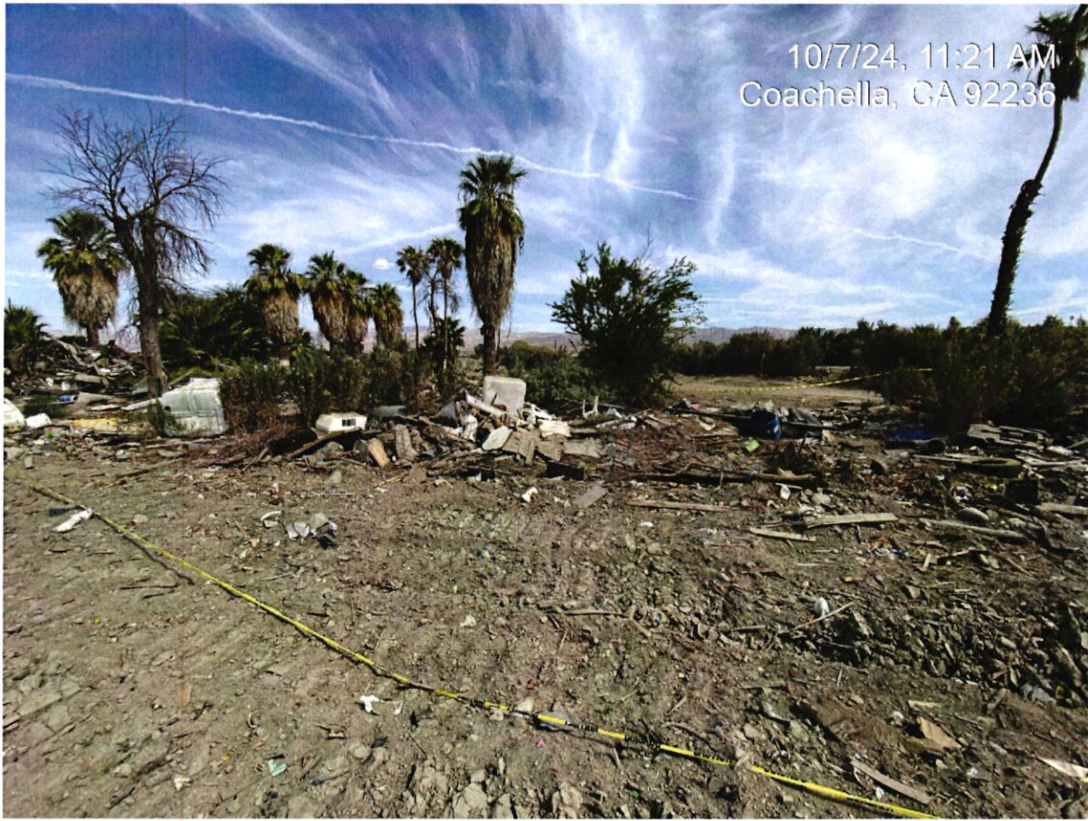
Debris field with positive Asbestos, northeast viewpoint of southeast area of Section F.
