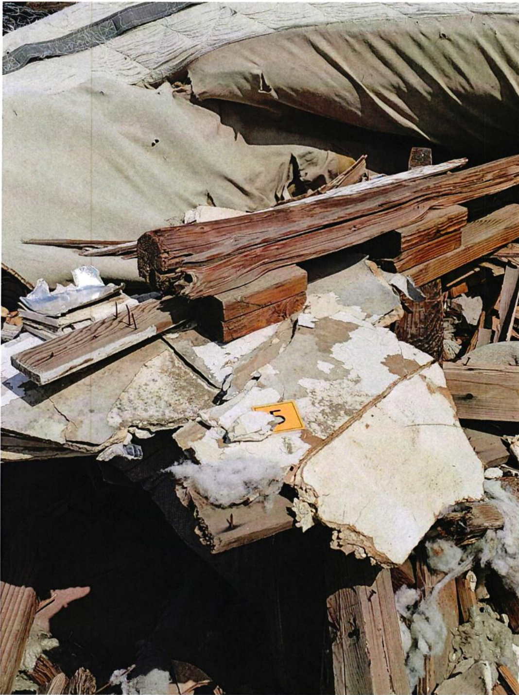
Photograph 9 – illustrates sample TE5 beige, joint compound from Zone E, asbestos present (3% Chrysotile).
