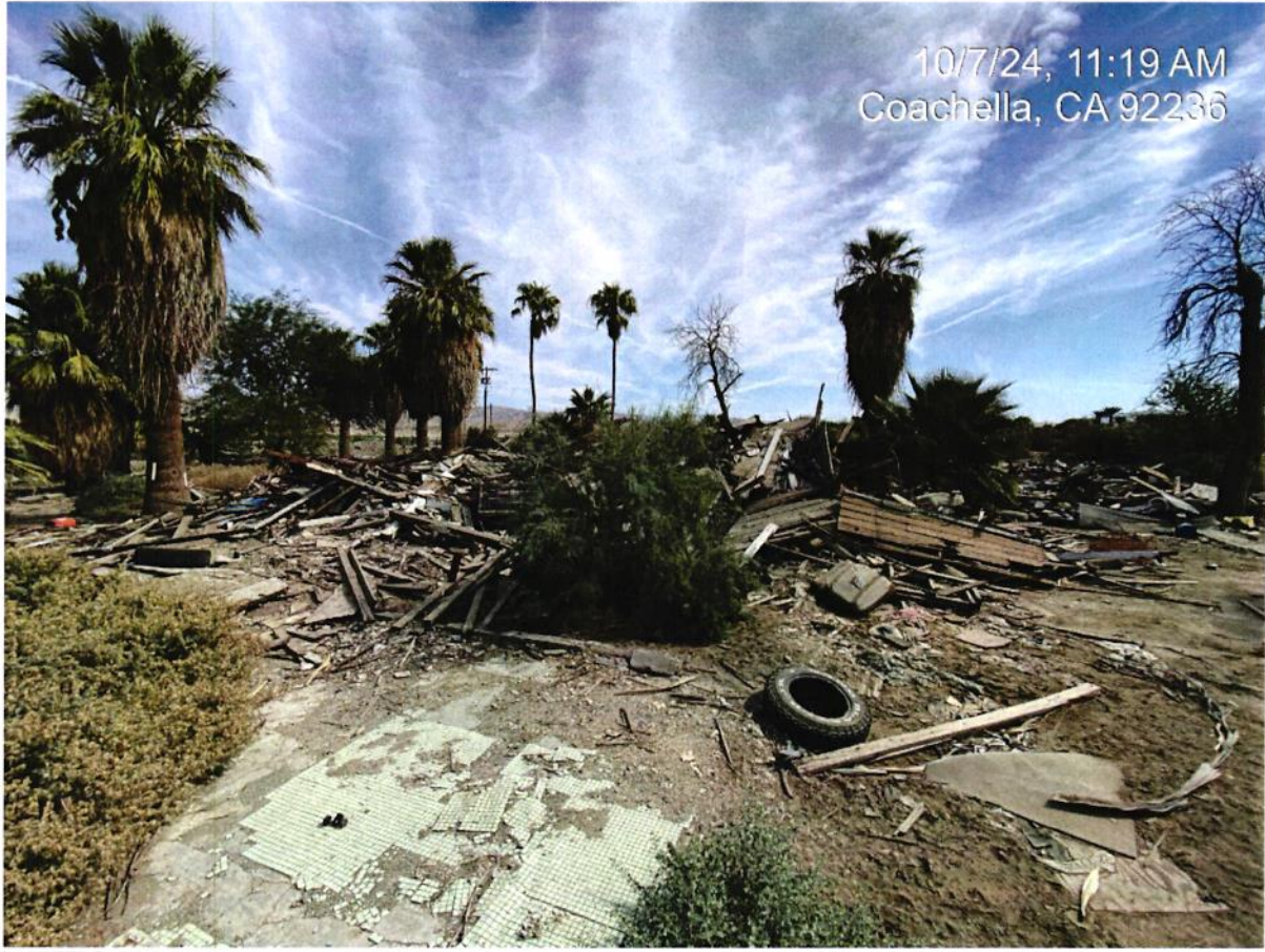
Debris field/demolished structure with positive Asbestos, northeast viewpoint of middle area of Section F.
