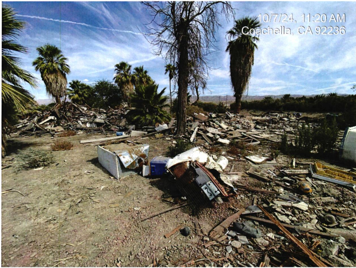
Debris field/demolished structure with positive Asbestos, north viewpoint of southeast area of Section F.
