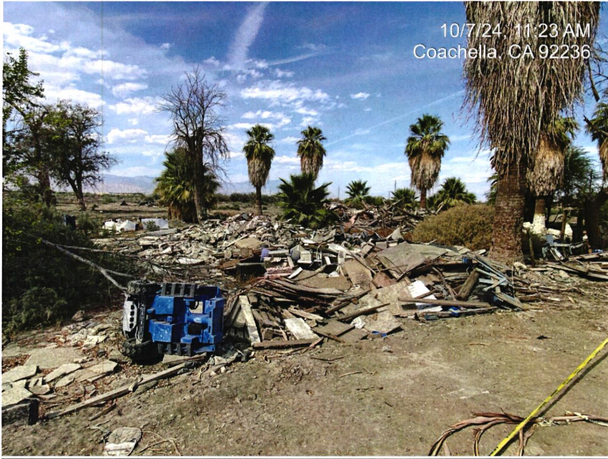
Debris field/demolished structure with positive Asbestos, west viewpoint of southeast corner of Section F.
