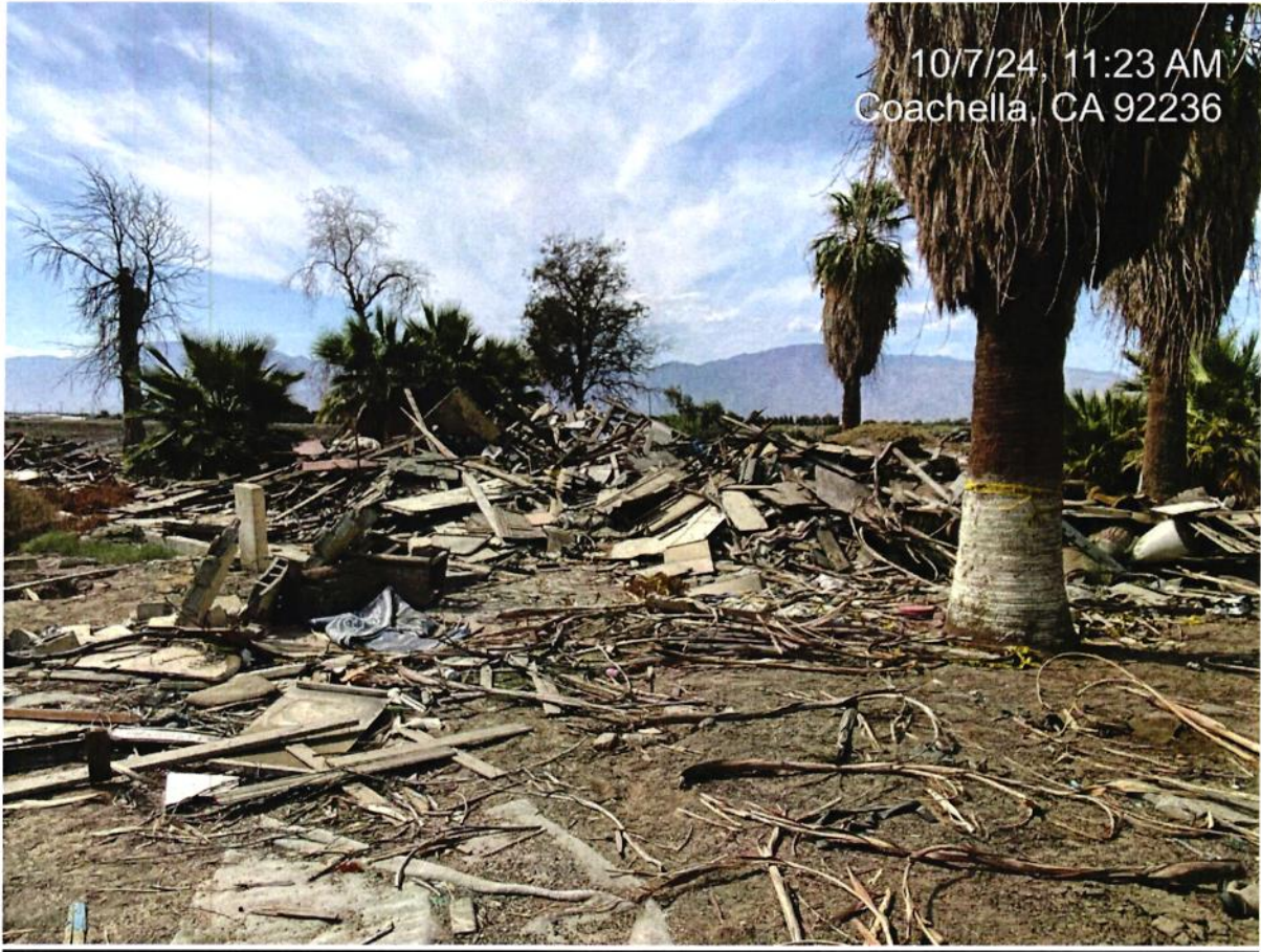
Debris pile (demolished structure) with positive Asbestos, south viewpoint of middle Section F.
