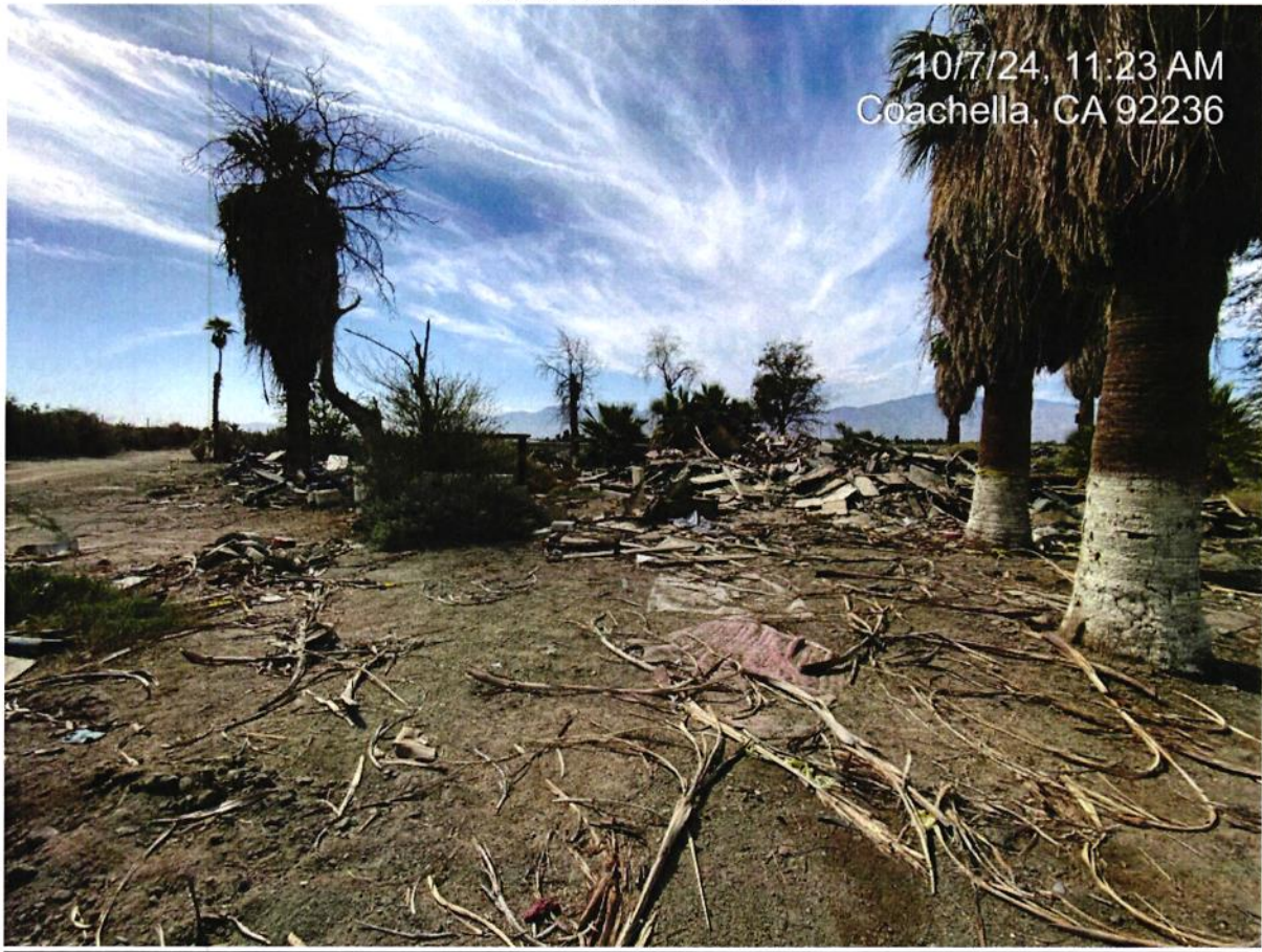
Debris field/demolished structure pile with positive Asbestos, south viewpoint of middle Section F.
