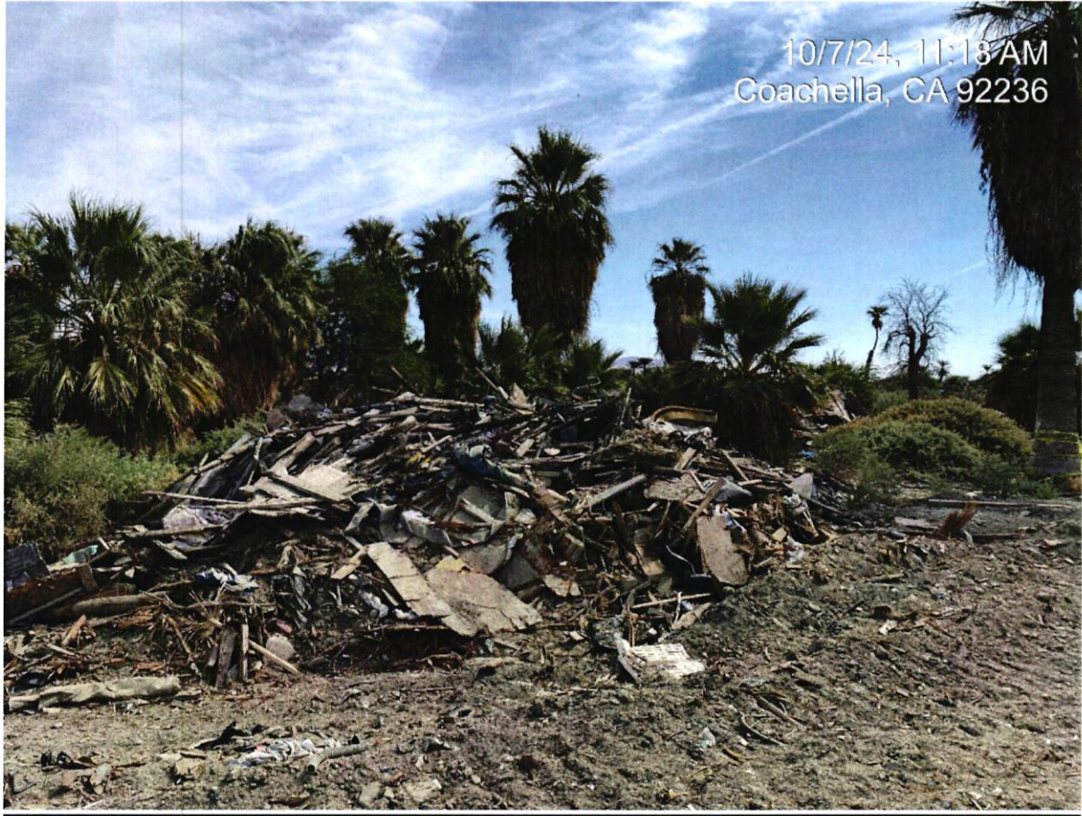
Debris field/demolished structure with positive Asbestos, east viewpoint of east side area of Section E.
