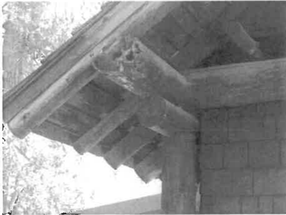
Photo 10- At the southeast corner the top beam of the wall has deteriorated due to moisture. Not an urgent matter but this should be repaired to keep water from continuing the deterioration.
