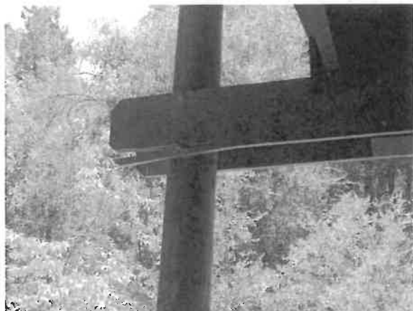
Photo 11- South side 2 X 12's spanning from posts to the beams have broken and may no longer be able to support the structure. The issue is that the bolts are too close to the boards' edge.
