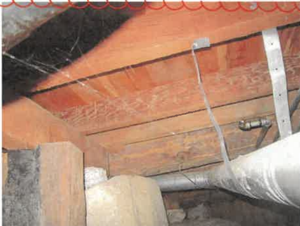
Photo 22- New floor framing of conventional sawn lumber at the east end of the basement.
