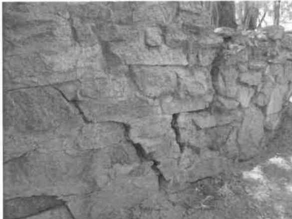
Photo 19- The retaining wall at the southeast corner of the building is failing. A tree, plus water flow, have contributed to this.
