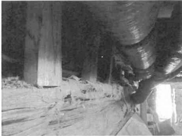
Photo 24 Cripple studs supporting the south wall and bearing on a rotted wall log. This is the cause of the floor sag in the southwest corner of the main room.
