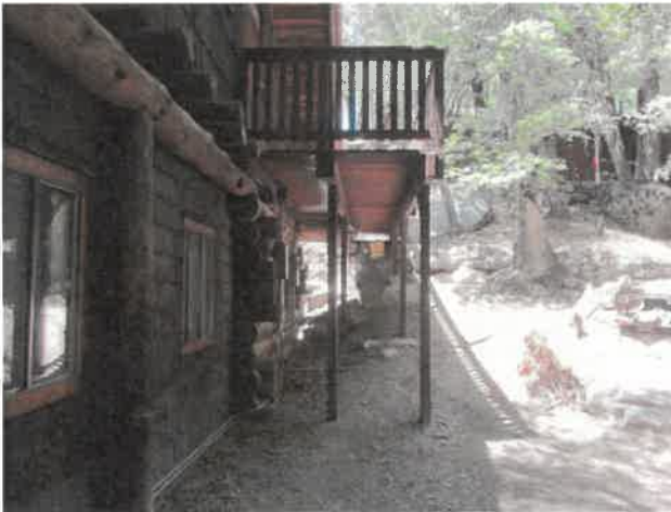
Photo 7 - East elevation and stairway. The stairway posts should have added "X" bracing for improved earthquake stability.
