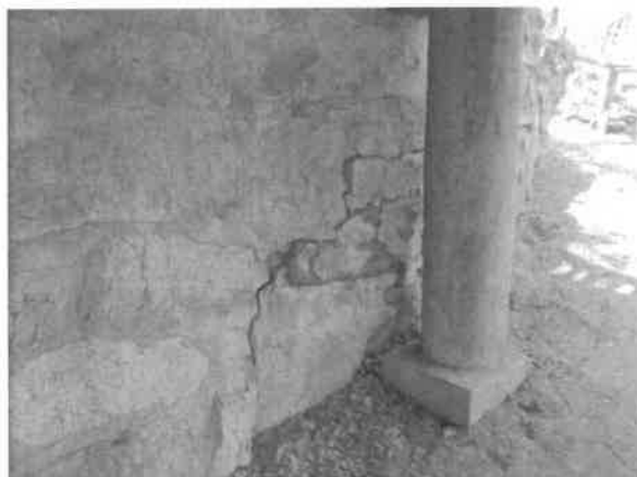
Photo 20- Another photo of the southeast corner showing how the retaining wall may eventually push against the building.
