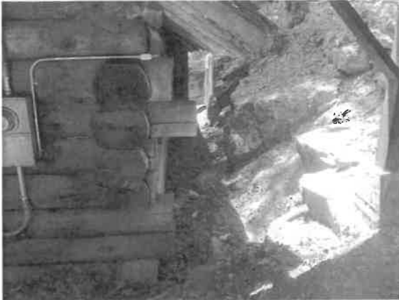
Photo 3 - North wall. Steep cut created for the building. Dirt and rocks fall down the hill to pile up against the building.
