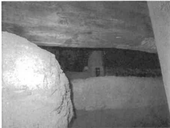
Photo 25- Basement showing an original support post. Many of these were removed for later construction.
