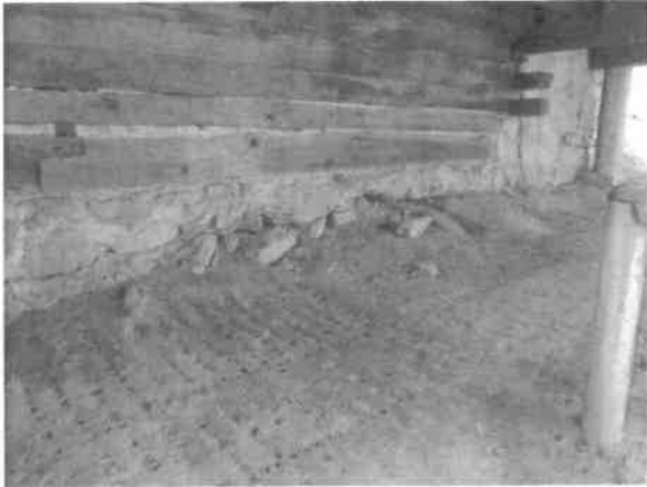
Photo 18- The foundation stones on part of the south side have failed and need to be reinstalled or a new segment of concrete foundation constructed.
