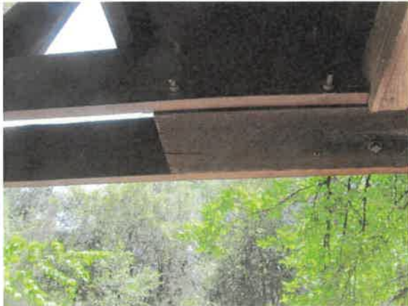
Photo 12- Another example of bolts being too close to the boards edge. This condition occurs in every beam to post connections
