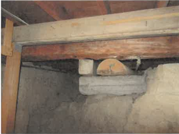
Photo 21- Basement view showing new framing and the original floor beam behind it. In many locations, the original beam is not supported.
