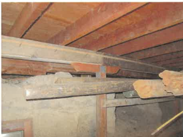
Photo 23- New and original floor beams shown. Note the notch in the original beam. It is not known whether this was original or notched for later construction access.
