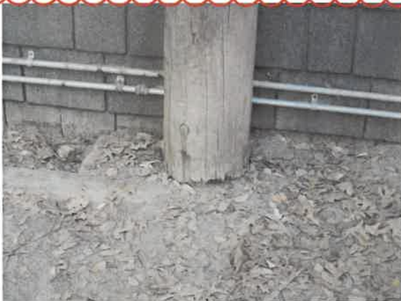
Photo 8 - Post on east side showing deterioration at base from water and snow. The post base should be kept clear of debris and dirt.
